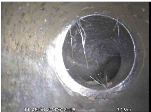
, 00:00:27, 3.17 m Crack, circumferential at joint from 1 o'clock to 9 o'clock
