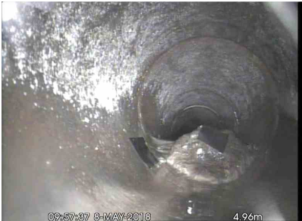
, 00:00:37, 4.96 m Settled deposits, hard or compacted at joint, 10% cross-sectional area loss
