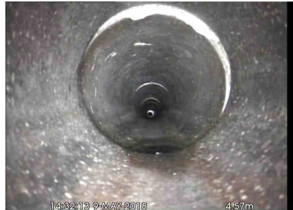
, 00:00:35, 4.57 m Attached deposits, other at joint from 11 o'clock to 2 o'clock, 5% cross-sectional area loss
