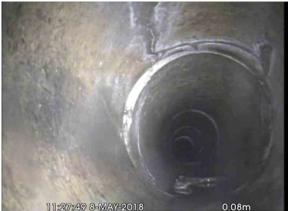
, 00:00:05, 0.08 m Crack, circumferential at joint from 7 o'clock to 1 o'clock
