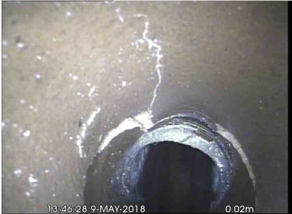
, 00:00:04, 0.02 m Broken pipe at joint from 9 o'clock to 4 o'clock ,
