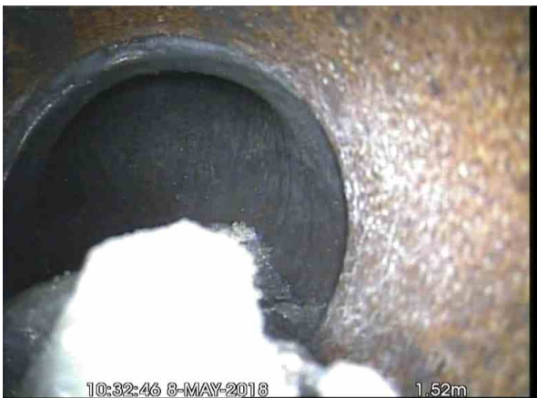
, 00:00:28, 1.52 m Finish node type, other special chamber, reference number: Downpipe
