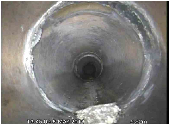
, 00:00:49, 5.62 m Attached deposits, other at joint from 12 o'clock to 12 o'clock, 5% cross-sectional area loss
