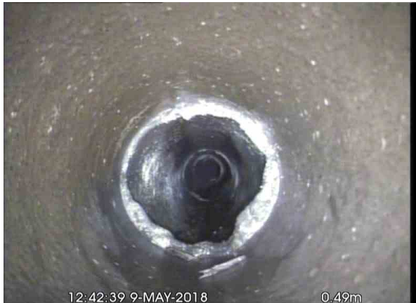
, 00:00:08, 0.49 m Attached deposits, other at joint from 12 o'clock to 12 o'clock, 5% cross-sectional area loss
