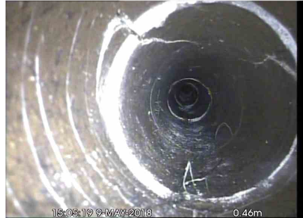
, 00:00:19, 0.46 m Fracture, circumferential at joint from 10 o'clock to 2 o'clock
