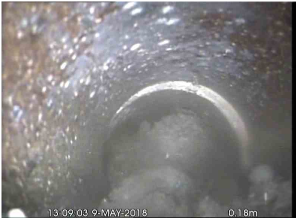
, 00:00:14, 0.18 m Settled deposits, fine, 90% cross-sectional area loss
