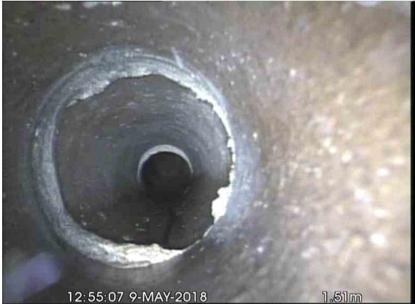
, 00:00:18, 1.51 m Attached deposits, other at joint from 5 o'clock to 3 o'clock, 5% cross-sectional area loss
