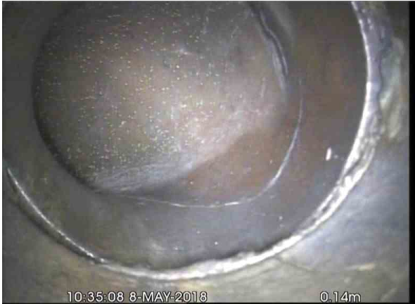
, 00:00:04, 0.14 m Crack, circumferential at joint from 12 o'clock to 7 o'clock
