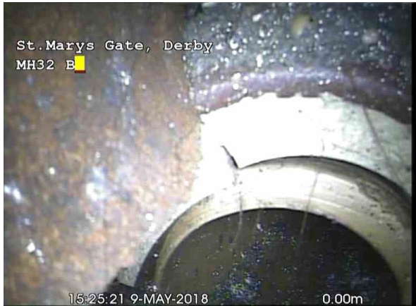
, 00:00:00, 0.15 m Joint displaced, large
