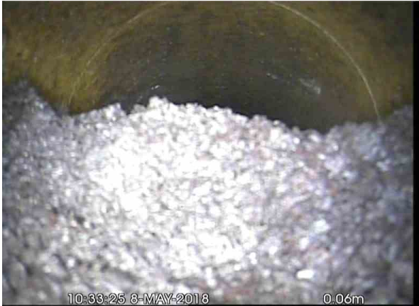
, 00:00:01, 0.06 m Settled deposits, fine, 40% cross-sectional area loss, start
