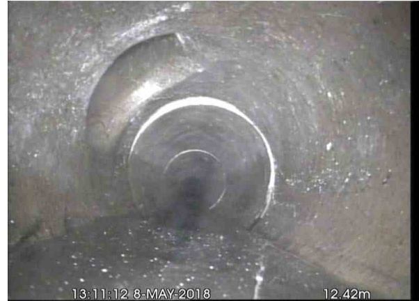
, 00:00:59, 12.42 m Junction at 10 o'clock, diameter: 100mm
