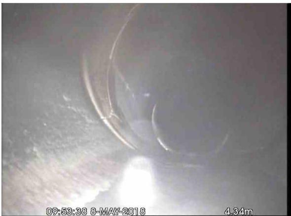
, 00:00:51, 4.34 m Crack, circumferential at joint from 7 o'clock to 12 o'clock
