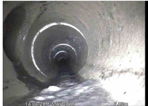
, 00:00:47, 7.03 m Junction at 10 o'clock, diameter: 100mm
