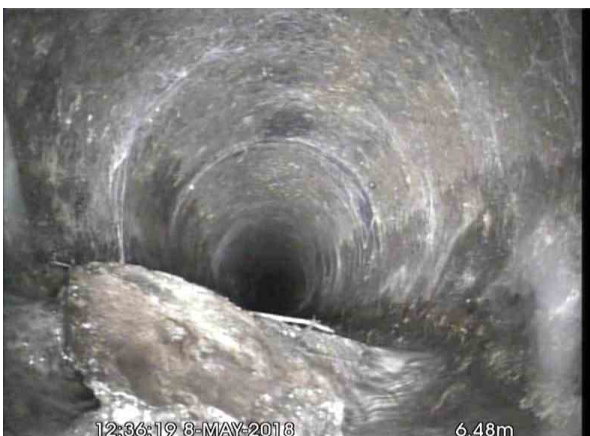
, 00:00:43, 6.48 m Settled deposits, other, 10% cross-sectional area loss
