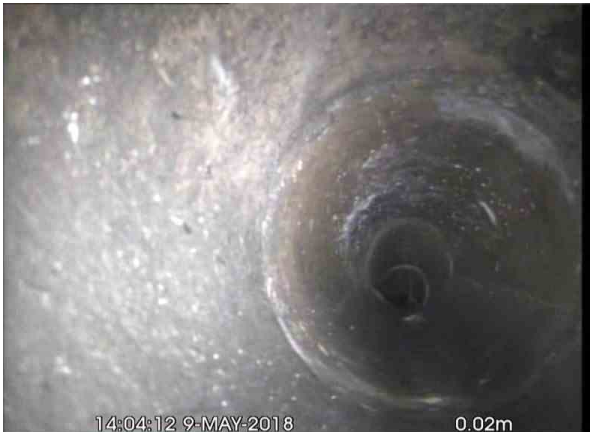
, 00:00:03, 0.02 m Crack, longitudinal at joint at 4 o'clock
