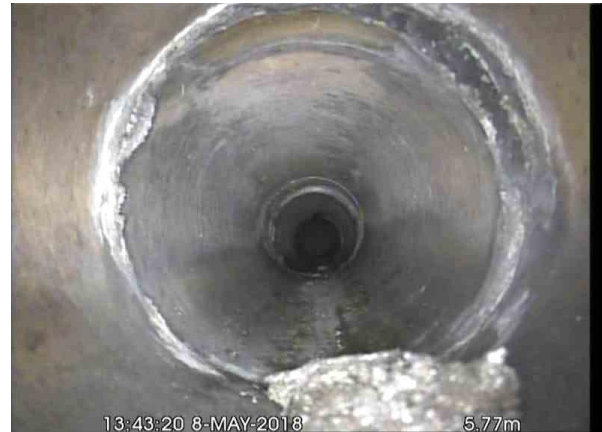
, 00:01:04, 5.77 m Crack, circumferential at joint from 11 o'clock to 1 o'clock
