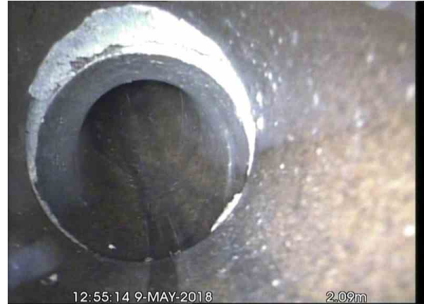
, 00:00:25, 2.09 m Joint displaced, medium
