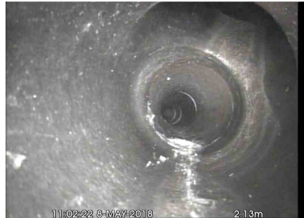
, 00:00:14, 2.13 m Junction at 1 o'clock, diameter: 100mm
