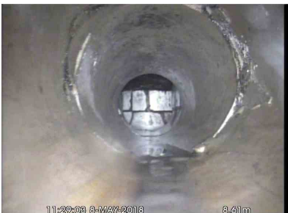
, 00:01:18, 8.61 m Cracks, multiple at joint from 11 o'clock to 4 o'clock
