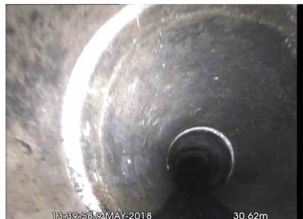
, 00:04:45, 30.54 m Crack, circumferential at joint from 7 o'clock to 2 o'clock
