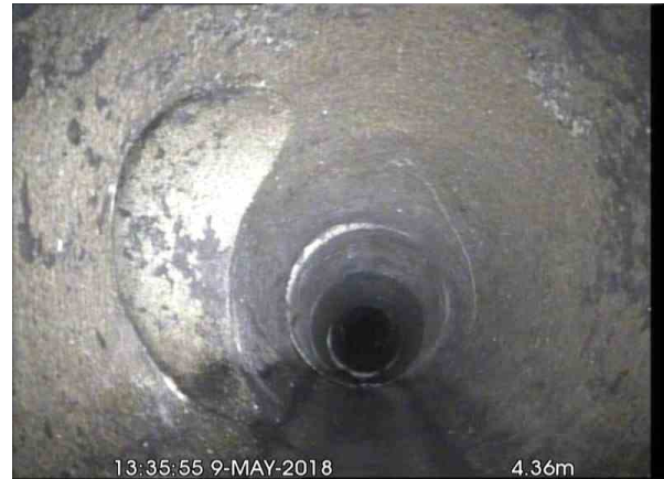
, 00:00:42, 4.36 m Junction at 9 o'clock, diameter: 100mm
