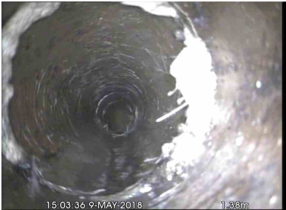
, 00:00:14, 1.38 m Attached deposits, encrustation at joint from 8 o'clock to 5 o'clock, 5% cross-sectional area loss
