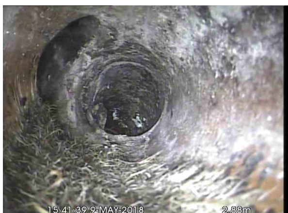
, 00:00:22, 2.88 m Roots, mass, 5% cross-sectional area loss
