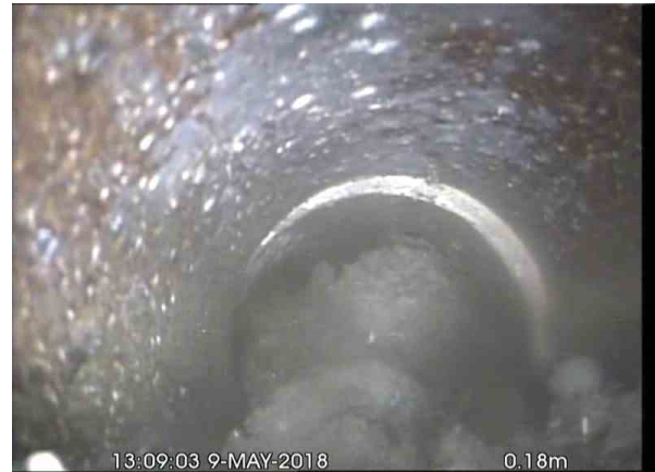
, 00:00:14, 0.18 m Survey abandoned, Unable to pass debris
