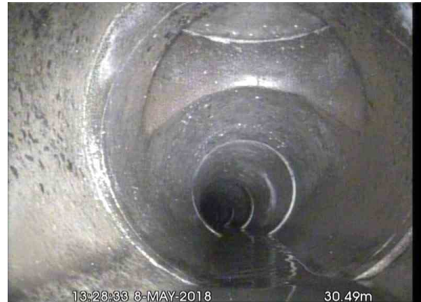
, 00:06:25, 30.49 m Crack, circumferential at joint from 12 o'clock to 12 o'clock
