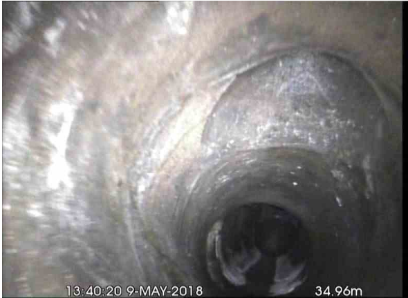
, 00:05:07, 34.96 m Junction at 1 o'clock, diameter: 100mm
