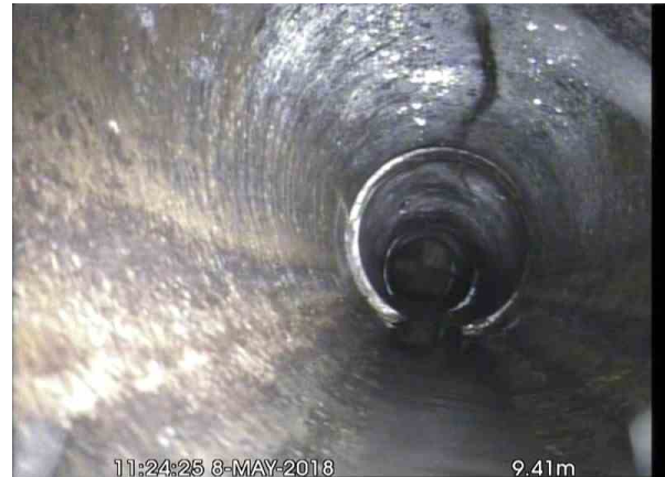
, 00:00:50, 9.41 m Crack, longitudinal at 12 o'clock
