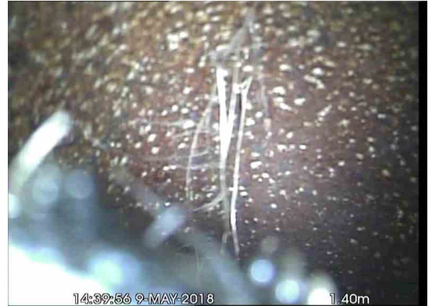
, 00:00:12, 1.40 m Finish node type, other special chamber, reference number: Downpipe
