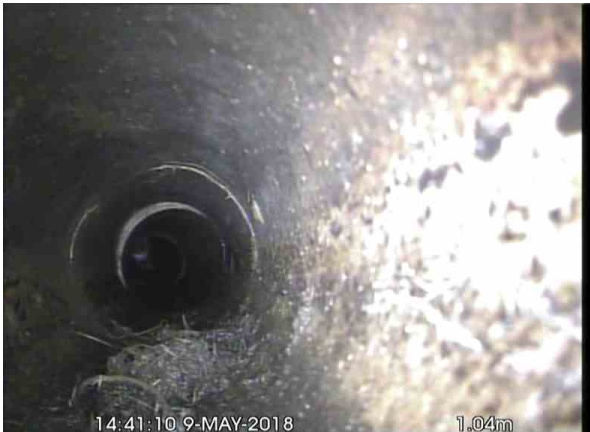
, 00:00:05, 1.04 m Roots, mass, 5% cross-sectional area loss
