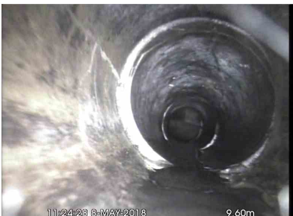
, 00:00:53, 9.60 m Crack, circumferential at joint from 10 o'clock to 3 o'clock
