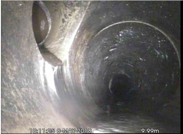
, 00:01:04, 9.99 m Junction at 9 o'clock, diameter: 100mm
