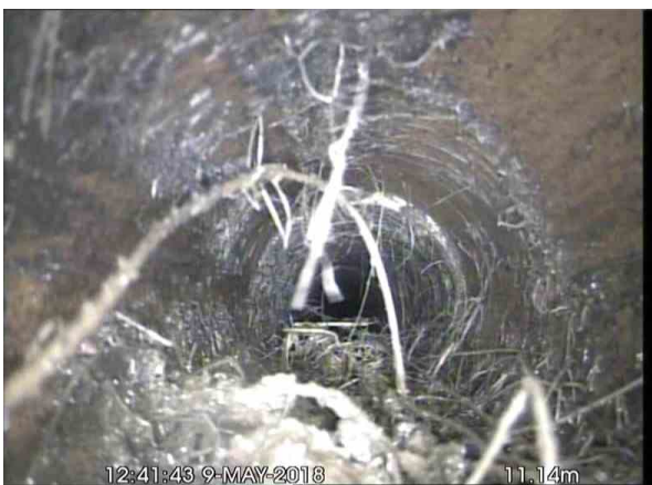
, 00:01:30, 11.14 m Survey abandoned, Unable to pass mass root ingress
