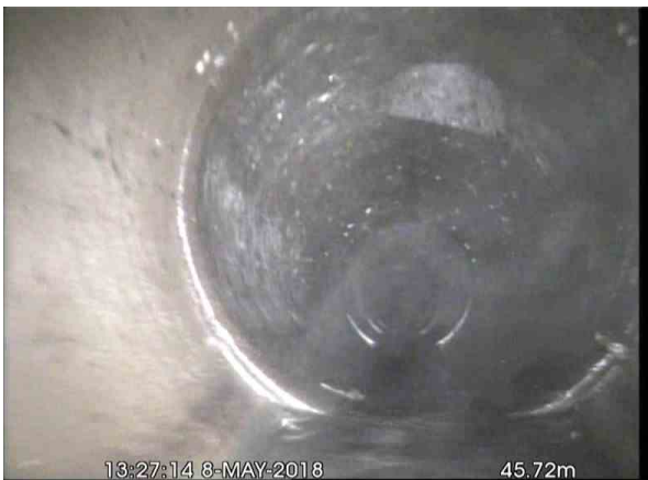
, 00:05:07, 45.72 m Junction at 1 o'clock, diameter: 100mm
