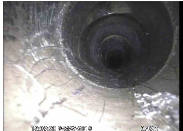
, 00:00:20, 3.49 m Junction at 11 o'clock, diameter: 100mm
