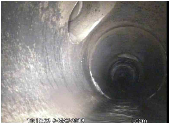
, 00:00:11, 1.02 m Junction at 10 o'clock, diameter: 100mm
