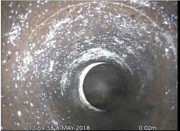
, 00:00:02, 0.02 m Crack, circumferential at joint from 9 o'clock to 3 o'clock
