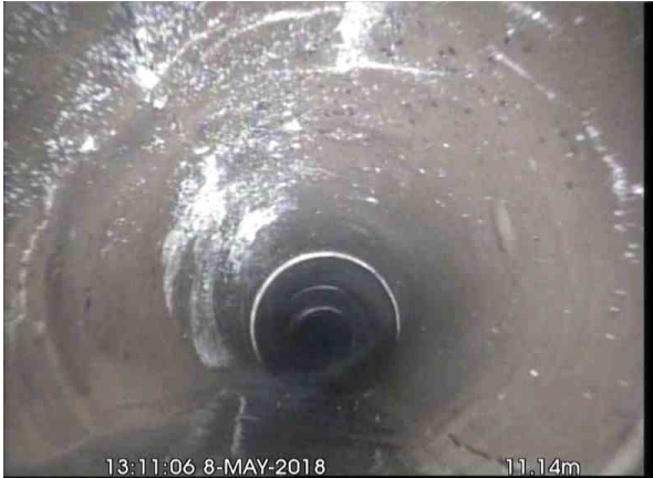
, 00:00:53, 11.14 m Crack, longitudinal at joint at 5 o'clock
