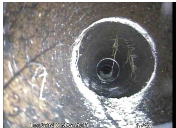
, 00:00:33, 1.74 m Roots, fine at joint
