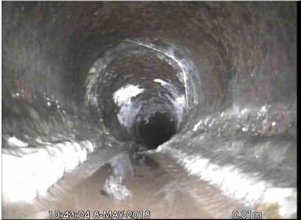
, 00:00:02, 0.01 m Attached deposits, grease from 4 o'clock to 8 o'clock, 5% cross-sectional area loss, start
