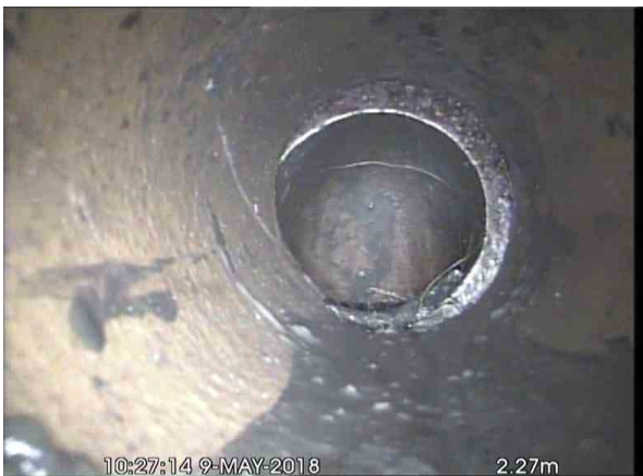
, 00:00:40, 2.39 m Joint displaced, medium
