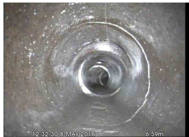
, 00:00:38, 6.59 m Crack, circumferential from 12 o'clock to 12 o'clock
