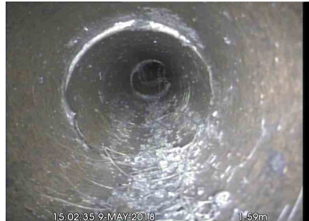
, 00:00:21, 1.59 m Settled deposits, fine, 15% cross-sectional area loss, finish
