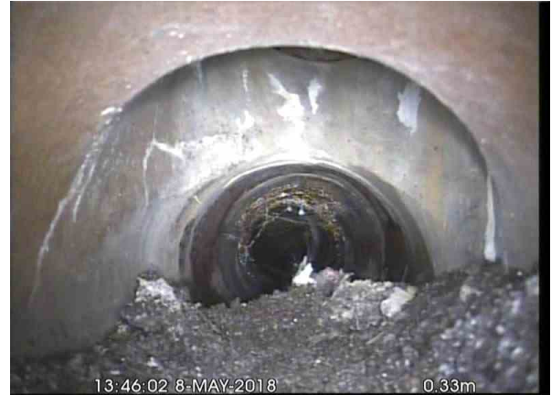
, 00:00:11, 0.33 m Settled deposits, fine, 25% cross-sectional area loss
