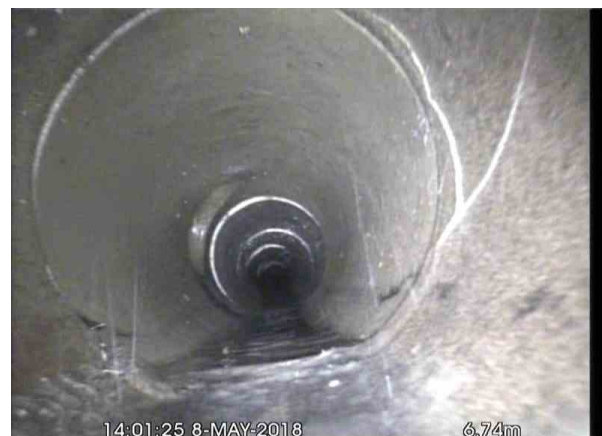
, 00:00:44, 6.74 m Crack, circumferential at joint from 1 o'clock to 4 o'clock
