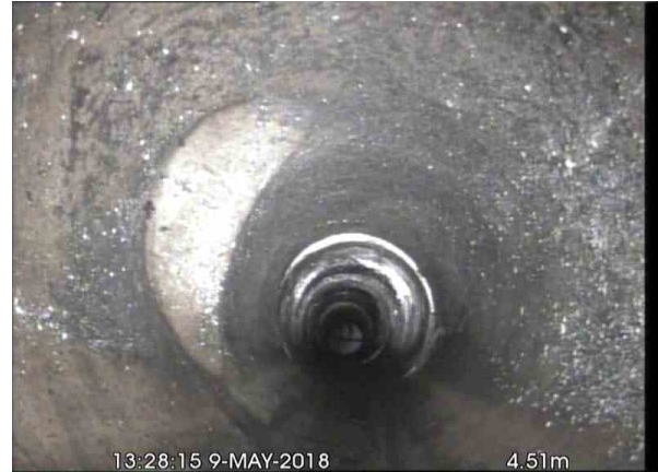
, 00:00:38, 4.51 m Junction at 10 o'clock, diameter: 100mm
