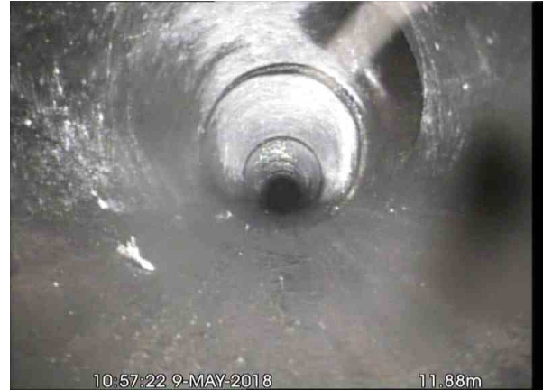
, 00:01:45, 11.88 m Junction at 2 o'clock, diameter: 100mm
