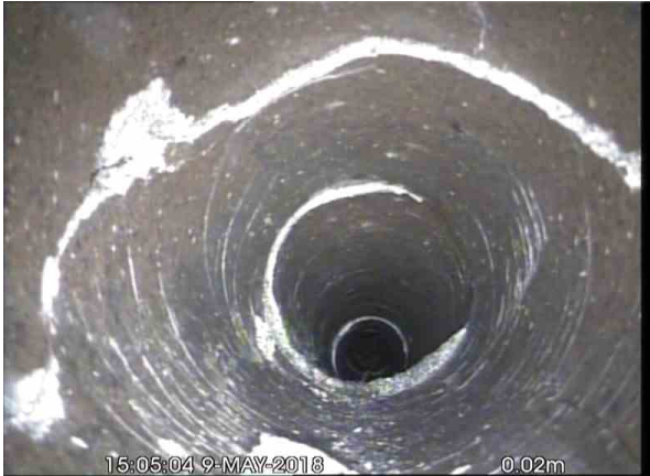
, 00:00:04, 0.02 m Fracture, circumferential at joint from 8 o'clock to 4 o'clock
