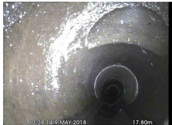
, 00:03:00, 17.80 m Junction at 1 o'clock, diameter: 100mm
