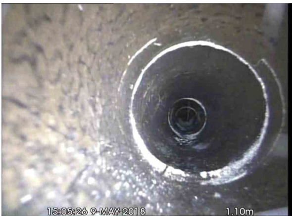
, 00:00:26, 1.10 m Crack, circumferential at joint from 1 o'clock to 11 o'clock
