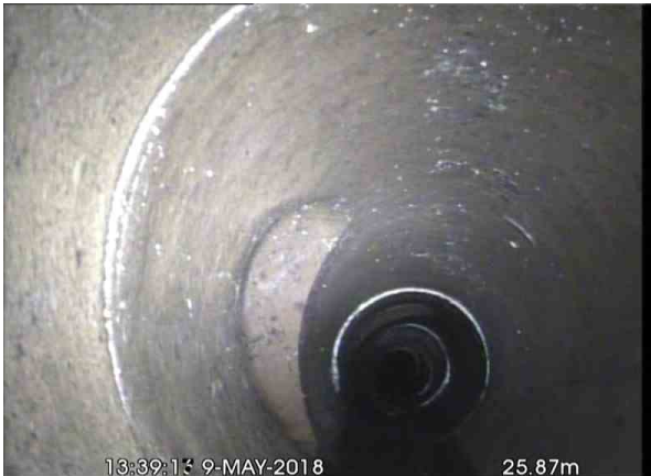
, 00:04:03, 25.87 m Junction at 9 o'clock, diameter: 100mm
