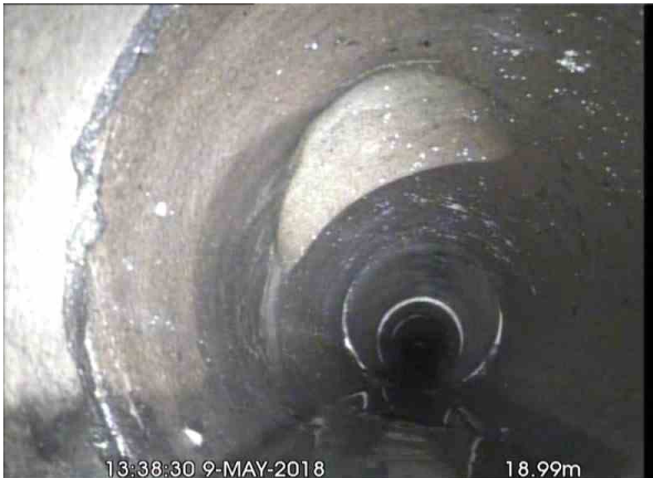
, 00:03:17, 18.99 m Junction at 11 o'clock, diameter: 100mm
