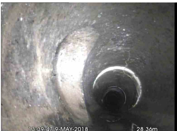
, 00:04:34, 28.36 m Junction at 9 o'clock, diameter: 100mm
