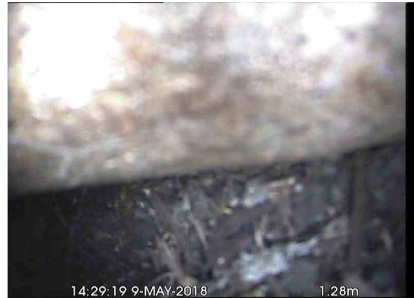
, 00:00:24, 1.28 m Finish node type, other special chamber, reference number: Downpipe
