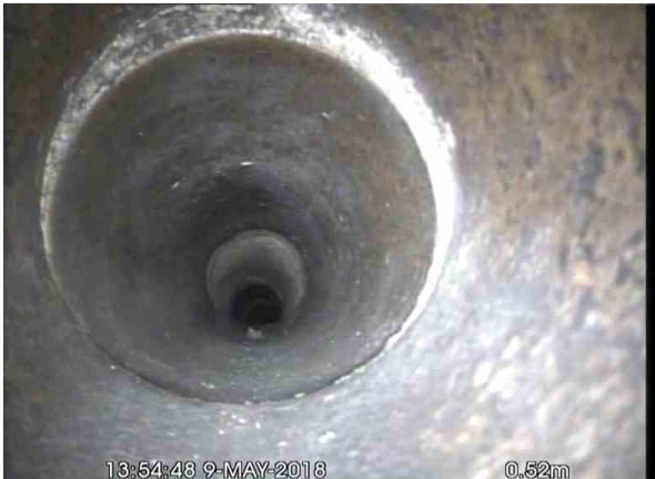
, 00:00:08, 0.52 m Joint displaced, medium
