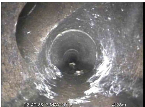
, 00:00:26, 4.26 m Junction at 10 o'clock, diameter: 100mm
