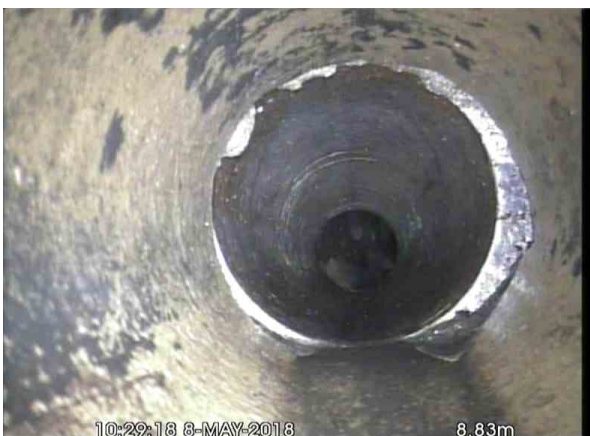
, 00:01:05, 8.83 m Joint displaced, medium
