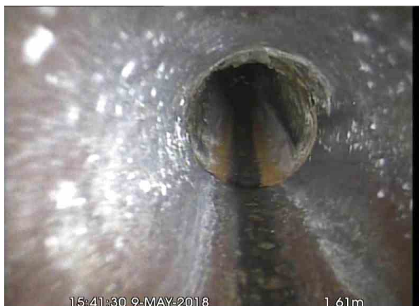
, 00:00:14, 1.61 m General remark, Sewer levels out at this point
