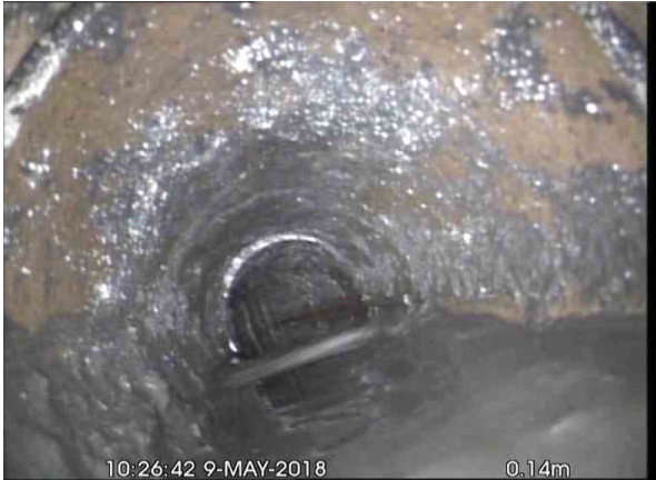
, 00:00:09, 0.14 m Settled deposits, fine, 10% cross-sectional area loss, start
