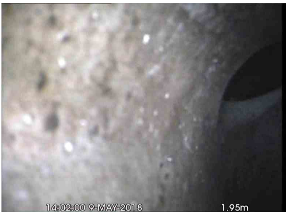
, 00:00:24, 1.95 m Finish node type, other special chamber, reference number: Downpipe
