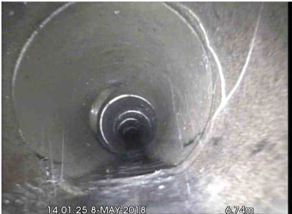
, 00:00:44, 6.74 m Roots, tap at joint
