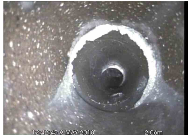
, 00:00:15, 2.06 m Attached deposits, other at joint from 8 o'clock to 5 o'clock, 5% cross-sectional area loss
