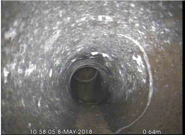
, 00:00:09, 0.64 m Crack, circumferential from 12 o'clock to 6 o'clock
