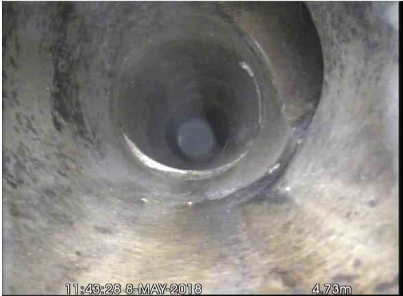
, 00:00:45, 4.73 m Junction at 2 o'clock, diameter: 100mm
