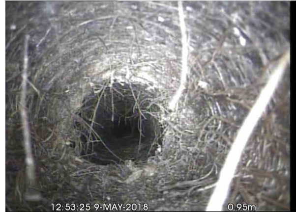
, 00:00:17, 0.95 m Survey abandoned, Unable to pass mass root ingress
