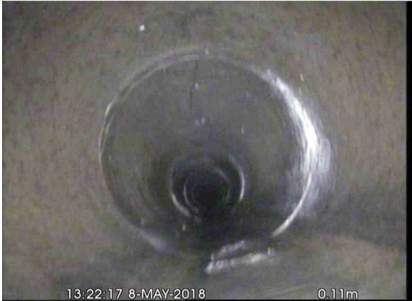
, 00:00:09, 0.11 m Crack, circumferential at joint from 9 o'clock to 1 o'clock
