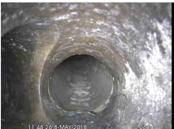
, 00:00:18, 1.90 m Crack, circumferential at joint from 3 o'clock to 9 o'clock
