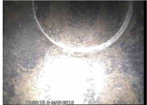
, 00:00:14, 1.27 m Finish node type, other special chamber, reference number: Vent pipe
