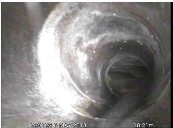
, 00:00:57, 10.21 m Crack, circumferential at joint from 12 o'clock to 9 o'clock
