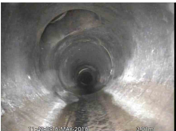
, 00:00:25, 3.01 m Junction at 11 o'clock, diameter: 100mm
