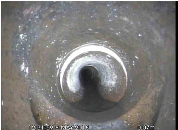
, 00:00:08, 0.07 m Junction at 6 o'clock, diameter: 150mm, External back drop
