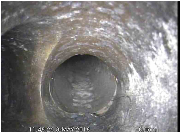
, 00:00:04, 0.06 m Junction at 9 o'clock, diameter: 100mm
