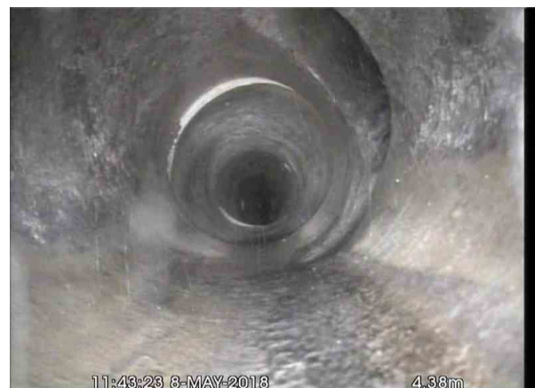
, 00:00:39, 4.40 m Junction at 1 o'clock, diameter: 100mm
