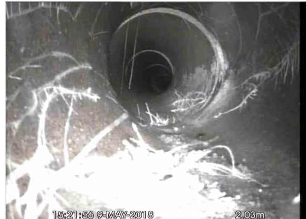
, 00:00:26, 2.03 m Roots, fine at joint
