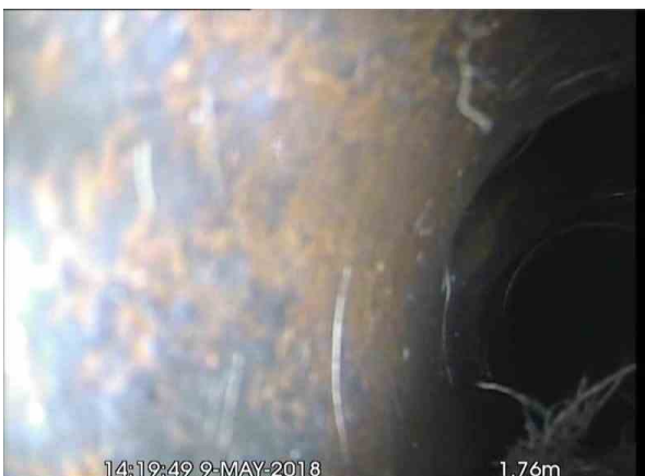
, 00:00:31, 1.76 m Junction at 10 o'clock, diameter: 100mm
