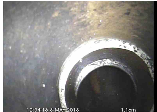
, 00:00:11, 1.16 m Joint displaced, medium
