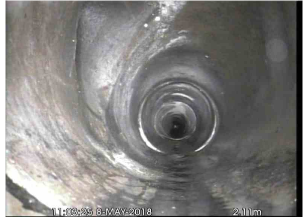
, 00:00:20, 2.11 m Junction at 10 o'clock, diameter: 100mm
