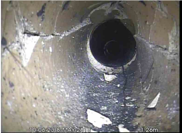
, 00:00:11, 1.26 m Broken pipe from 9 o'clock to 3 o'clock
