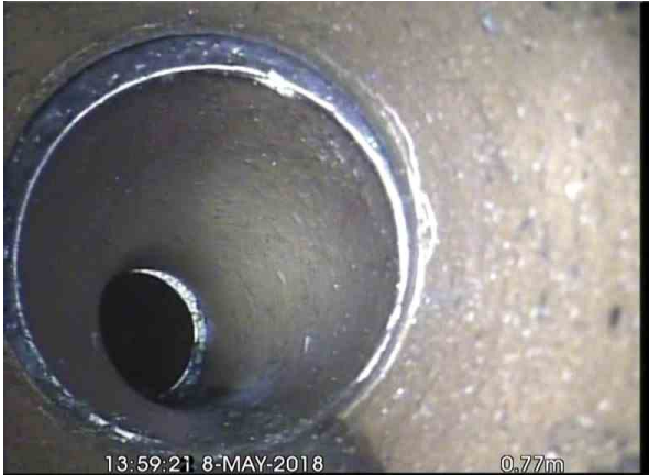
, 00:00:11, 0.77 m Joint displaced, medium
