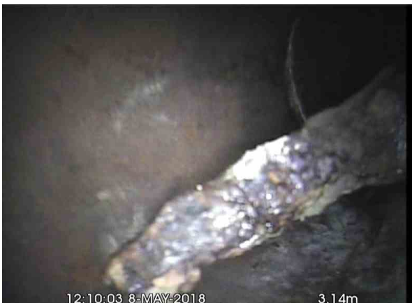
, 00:00:36, 3.14 m Other obstacles from 3 o'clock to 7 o'clock, 30% cross-sectional area loss
