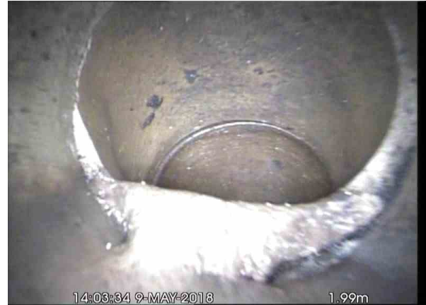
, 00:00:17, 1.99 m Attached deposits, other at joint from 5 o'clock to 7 o'clock, 5% cross-sectional area loss
