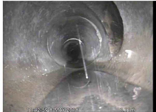
, 00:00:16, 1.11 m Junction at 2 o'clock, diameter: 100mm
