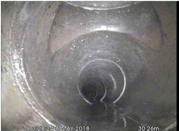
, 00:06:16, 30.26 m Junction at 12 o'clock, diameter: 150mm
