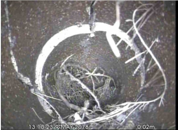
, 00:00:17, 0.02 m Fracture, multiple at joint from 7 o'clock to 1 o'clock
