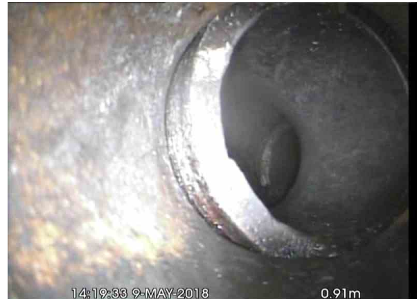
, 00:00:15, 0.90 m Joint displaced, medium
