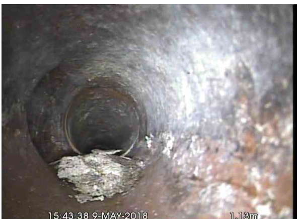
, 00:00:13, 1.13 m Settled deposits, other at joint, 5% cross-sectional area loss
