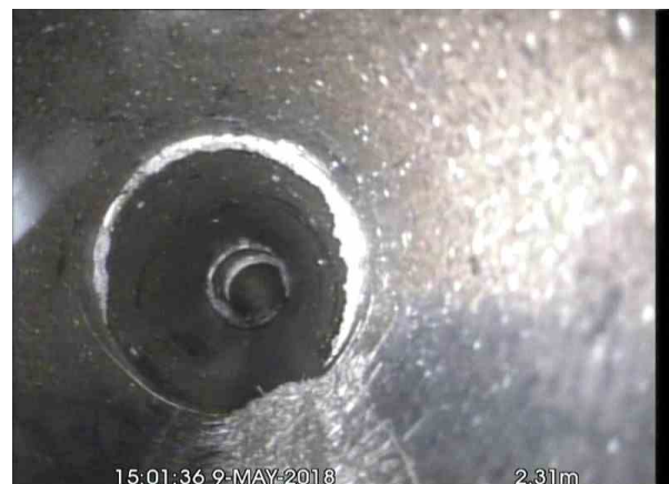
, 00:00:22, 2.31 m Crack, circumferential at joint from 4 o'clock to 8 o'clock
