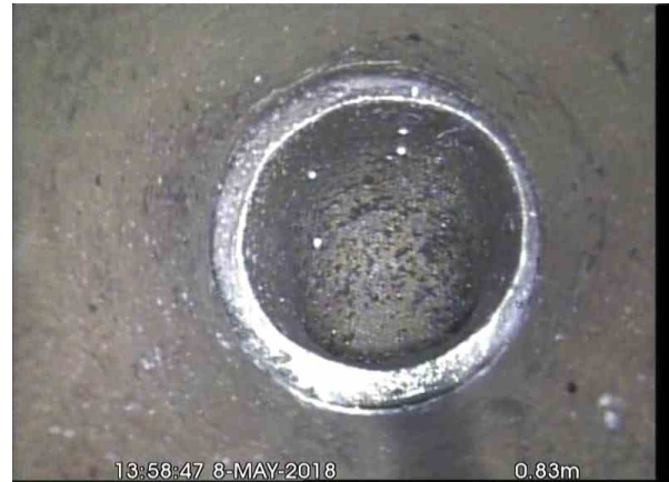
, 00:00:13, 0.83 m Joint displaced, medium
