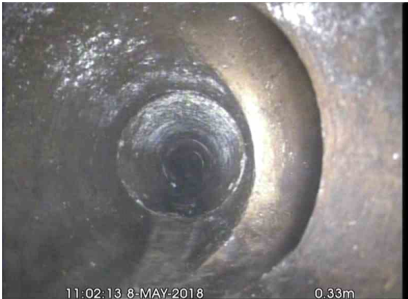
, 00:00:05, 0.33 m Junction at 3 o'clock, diameter: 100mm
