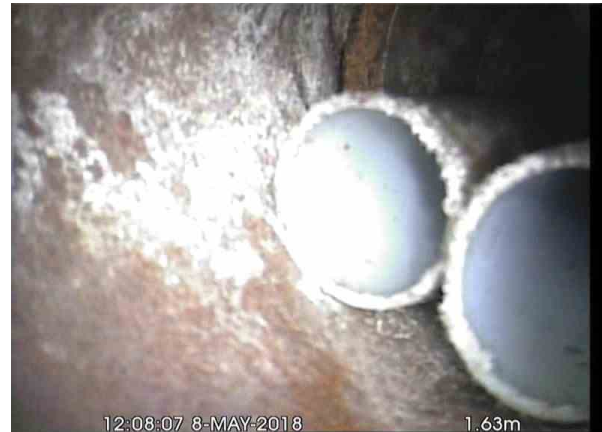
, 00:00:25, 1.63 m Other obstacles in invert from 4 o'clock to 8 o'clock, 25% cross-sectional area loss
