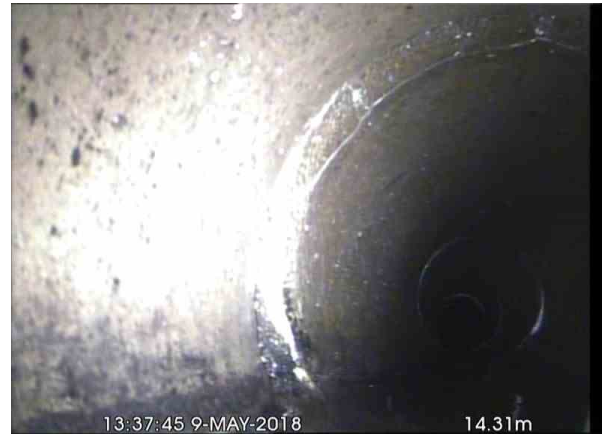
, 00:02:32, 14.31 m Crack, circumferential at joint from 7 o'clock to 1 o'clock
