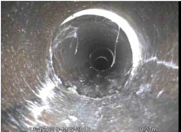
, 00:00:05, 0.27 m Joint displaced, medium
