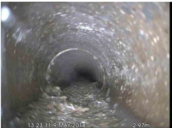
, 00:00:37, 2.97 m Settled deposits, fine, 15% cross-sectional area loss, start
