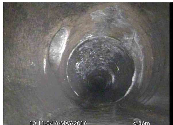
, 00:00:43, 6.86 m Junction at 10 o'clock, diameter: 100mm
