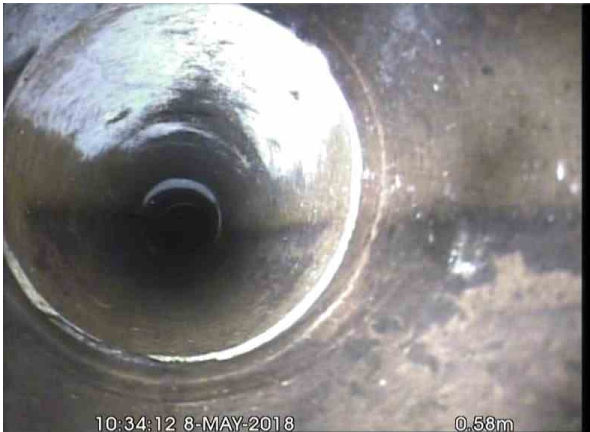
, 00:00:09, 0.58 m Crack, circumferential at joint from 12 o'clock to 12 o'clock
