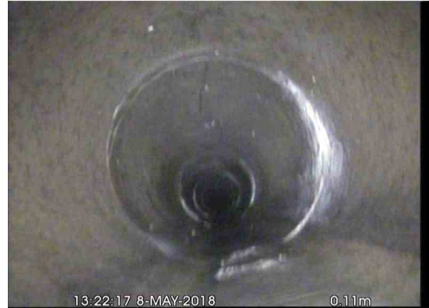
, 00:00:09, 0.11 m Crack, longitudinal at joint at 12 o'clock
