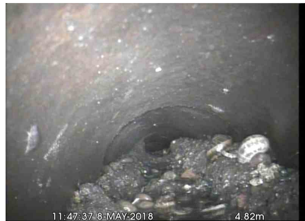
, 00:00:43, 4.82 m Settled deposits, coarse at joint, 75% cross-sectional area loss
