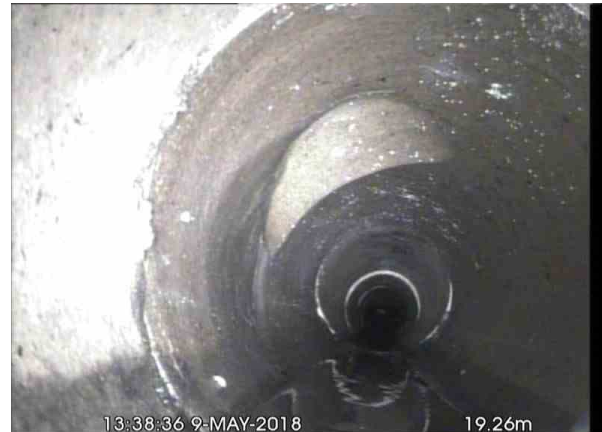
, 00:03:23, 19.26 m Junction at 11 o'clock, diameter: 100mm
