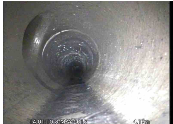
, 00:00:29, 4.17 m Junction at 10 o'clock, diameter: 100mm
