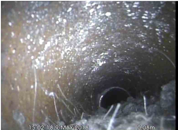
, 00:00:03, 0.02 m Settled deposits, fine, 15% cross-sectional area loss, start
