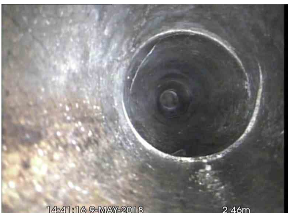
, 00:00:12, 2.46 m Crack, circumferential at joint from 12 o'clock to 12 o'clock
