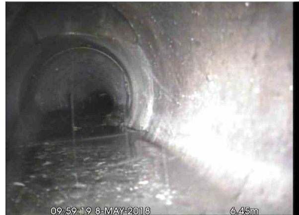
, 00:02:19, 6.45 m Junction at 1 o'clock, diameter: 100mm
