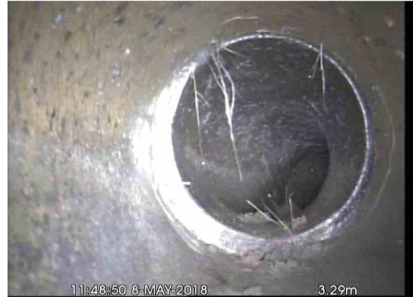
, 00:00:27, 3.17 m Roots, fine at joint
