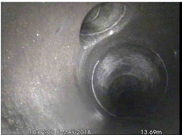
, 00:01:39, 13.69 m Junction at 11 o'clock, diameter: 100mm
