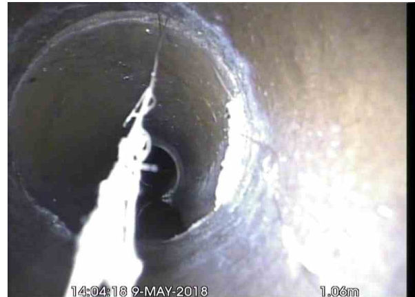
, 00:00:09, 1.06 m Roots, tap at joint
