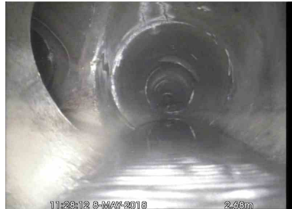
, 00:00:28, 2.68 m Junction at 9 o'clock, diameter: 100mm
