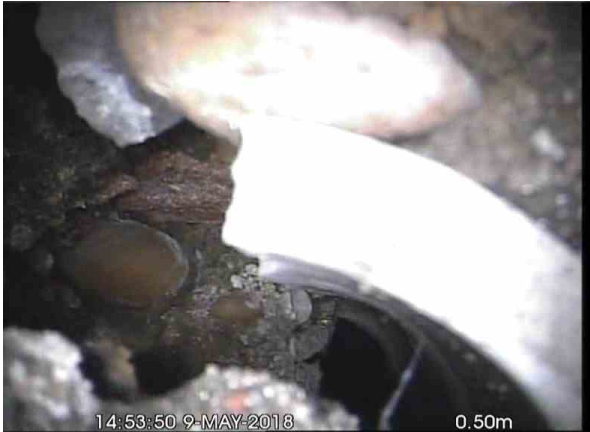
, 00:00:10, 0.50 m Collapsed drain or sewer
