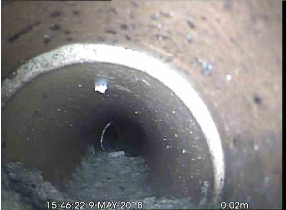
, 00:00:03, 0.02 m Settled deposits, fine, 5% cross-sectional area loss, start
