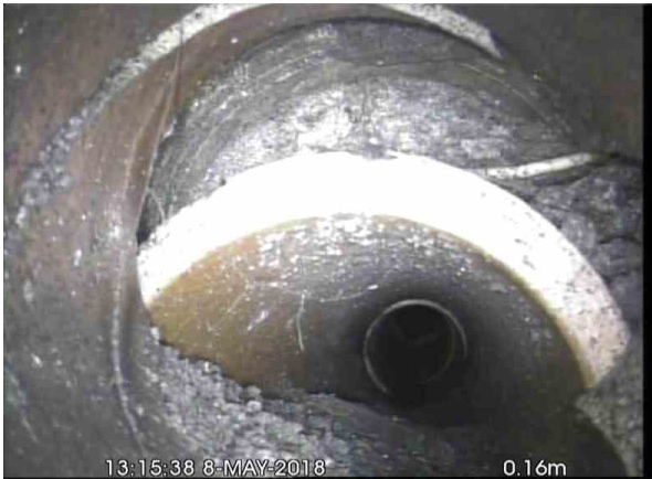
, 00:00:20, 0.16 m Collapsed drain or sewer
