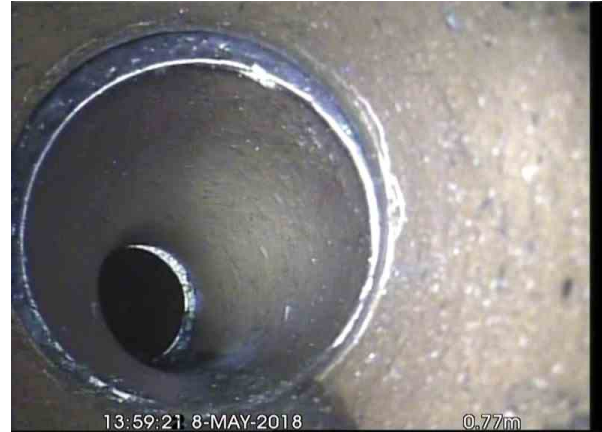
, 00:00:11, 0.77 m Crack, circumferential at joint from 1 o'clock to 6 o'clock
