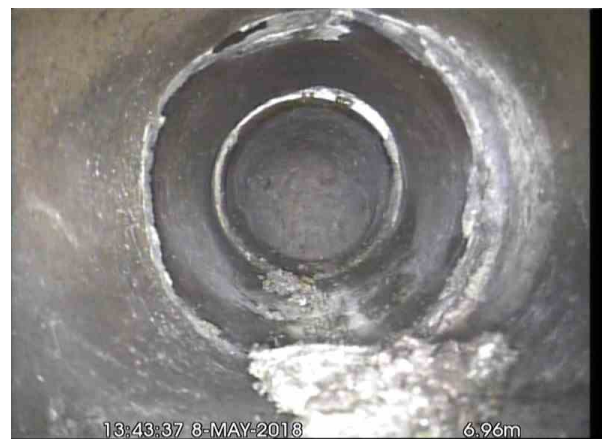
, 00:01:20, 6.96 m Settled deposits, other at joint, 5% cross-sectional area loss
