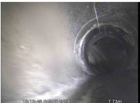
, 00:00:34, 7.73 m Crack, circumferential at joint from 7 o'clock to 4 o'clock
