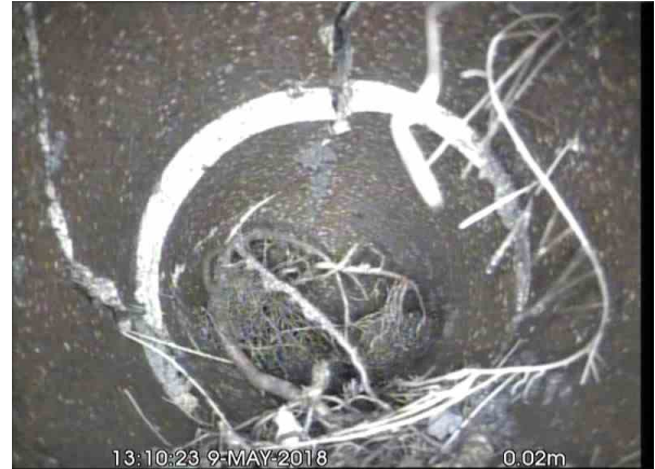
, 00:00:17, 0.02 m Roots, mass at joint, 20% cross-sectional area loss
