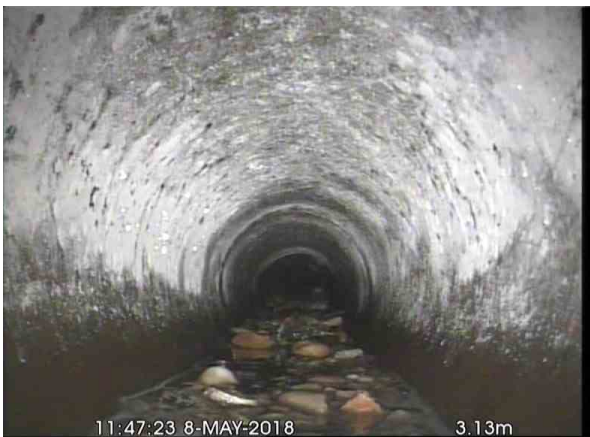
, 00:00:29, 3.13 m Settled deposits, coarse at joint, 10% cross-sectional area loss
