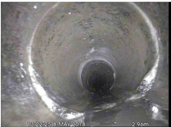
, 00:00:17, 2.96 m Attached deposits, other at joint from 4 o'clock to 8 o'clock, 5% cross-sectional area loss
