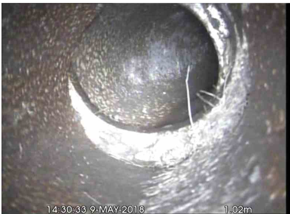
, 00:00:27, 1.02 m Joint displaced, medium
