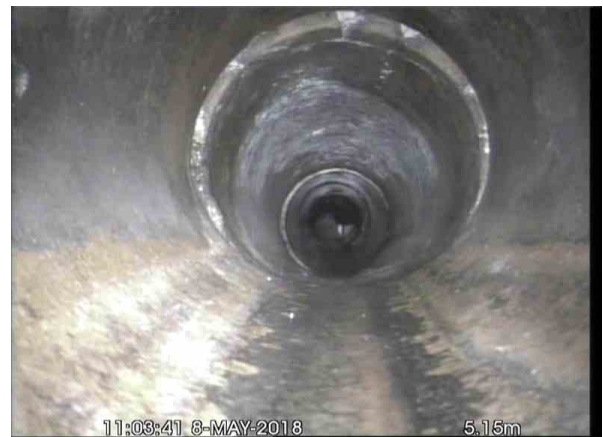
, 00:00:36, 5.15 m Crack, circumferential at joint from 11 o'clock to 2 o'clock
