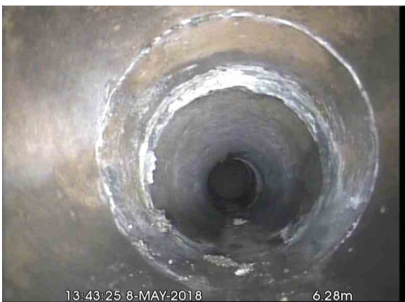
, 00:01:09, 6.28 m Crack, circumferential at joint from 12 o'clock to 12 o'clock
