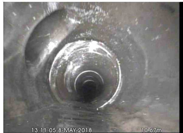
, 00:00:52, 10.67 m Junction at 10 o'clock, diameter: 100mm
