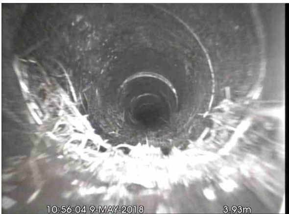
, 00:00:27, 3.93 m Crack, circumferential at joint from 11 o'clock to 6 o'clock
