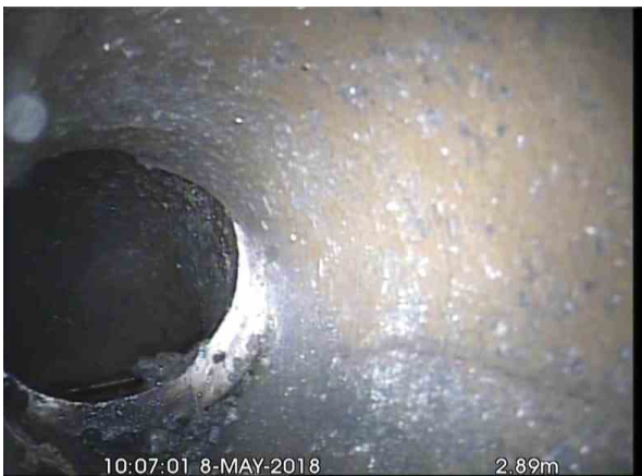
, 00:00:49, 2.89 m Joint displaced, medium
