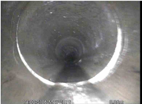
, 00:00:10, 0.06 m Crack, circumferential at joint from 1 o'clock to 5 o'clock
