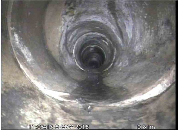
, 00:00:08, 0.81 m Junction at 9 o'clock, diameter: 100mm
