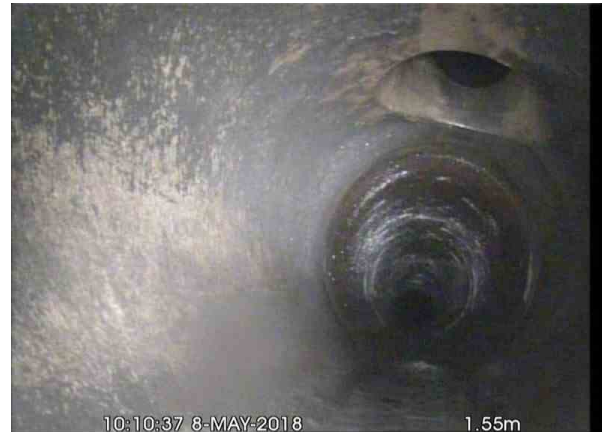
, 00:00:16, 1.51 m Junction at 1 o'clock, diameter: 100mm
