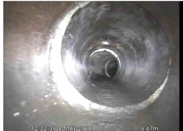
, 00:00:47, 6.67 m Joint displaced, medium
