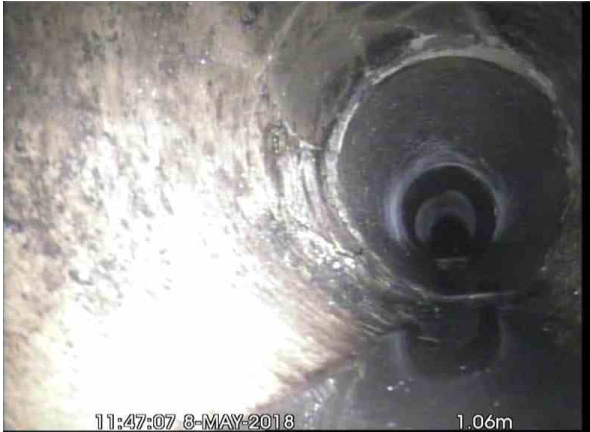
, 00:00:13, 1.06 m Fracture, multiple at joint from 12 o'clock to 12 o'clock
