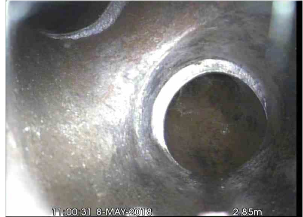
, 00:00:24, 2.58 m Junction at 10 o'clock, diameter: 100mm
