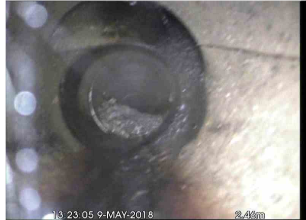
, 00:00:31, 2.46 m Junction at 1 o'clock, diameter: 100mm
