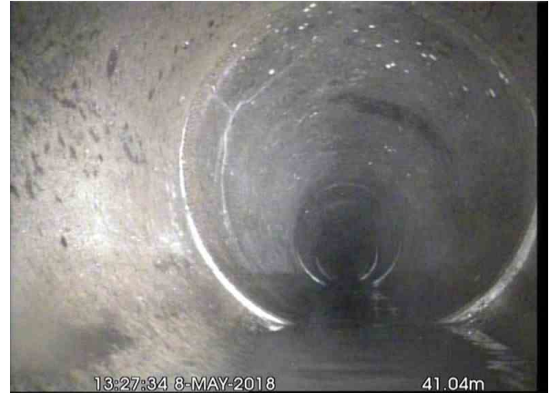
, 00:05:26, 41.04 m Crack, circumferential at joint from 8 o'clock to 11 o'clock
