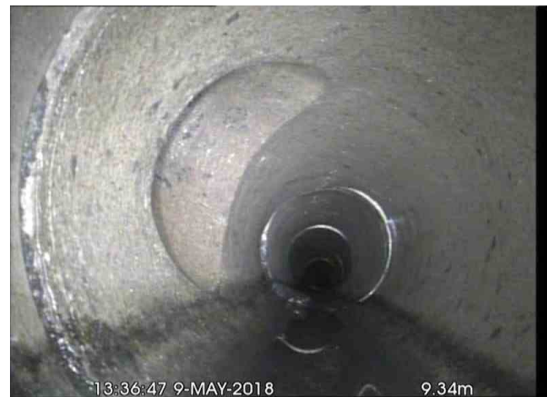
, 00:01:34, 9.34 m Junction at 10 o'clock, diameter: 100mm
