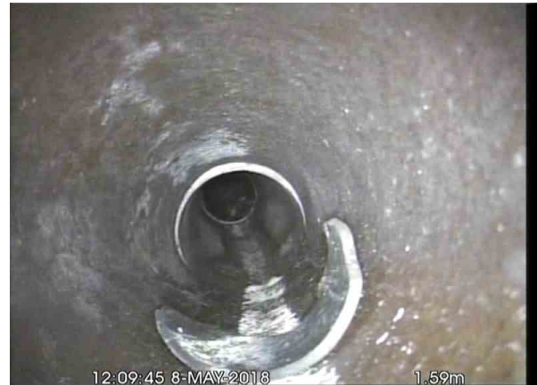
, 00:00:18, 1.59 m Obstacles, pipe material in invert from 4 o'clock to 7 o'clock, 5% cross-sectional area loss
