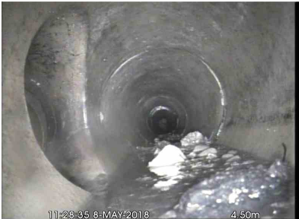
, 00:00:51, 4.50 m Settled deposits, fine, 5% cross-sectional area loss
