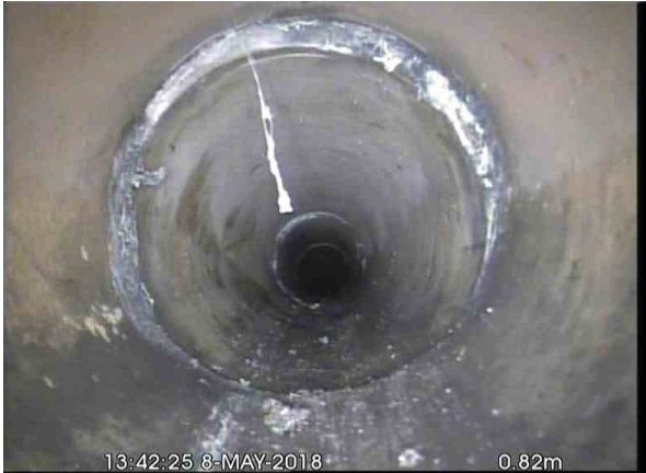
, 00:00:09, 0.82 m Joint displaced, medium
