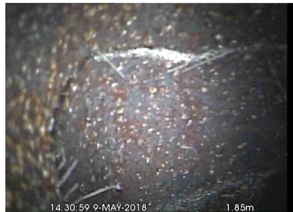
, 00:00:53, 1.85 m Finish node type, other special chamber, reference number: Downpipe
