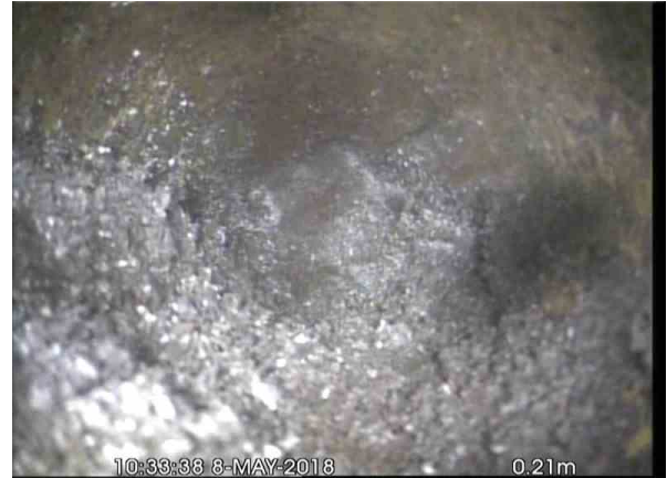
, 00:00:15, 0.21 m Survey abandoned, Unable to pass debris
