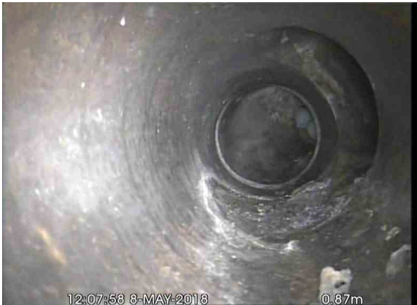
, 00:00:16, 0.87 m Junction at 2 o'clock, diameter: 100mm
