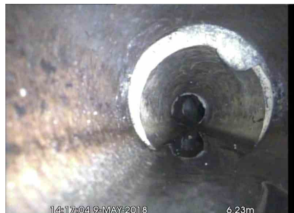
, 00:01:20, 6.23 m Attached deposits, other at joint from 12 o'clock to 2 o'clock, 5% cross-sectional area loss
