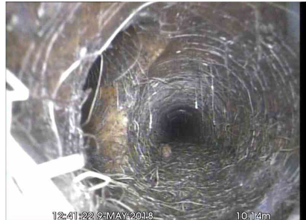
, 00:01:09, 10.14 m Junction at 10 o'clock, diameter: 100mm
