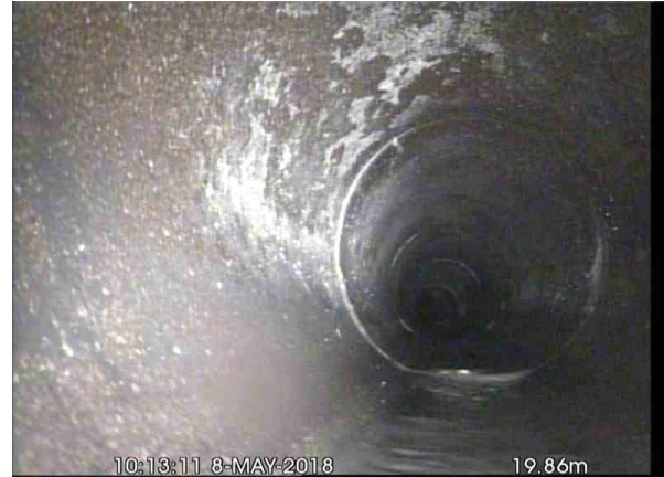
, 00:02:49, 19.86 m Survey abandoned, Unable to push camera any further
