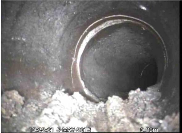
, 00:00:03, 0.02 m Crack, circumferential at joint from 12 o'clock to 12 o'clock
