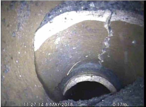
, 00:00:06, 0.17 m Broken pipe from 10 o'clock to 2 o'clock
