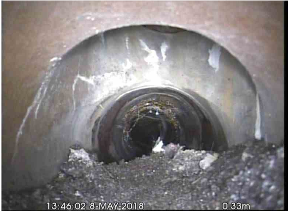
, 00:00:11, 0.33 m Junction at 12 o'clock, diameter: 100mm
