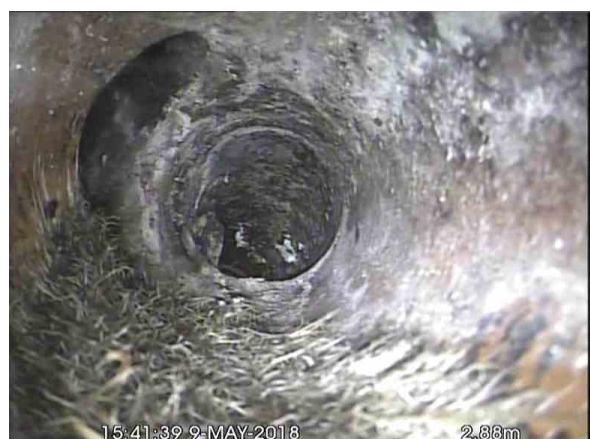
, 00:00:22, 2.88 m Junction at 10 o'clock, diameter: 100mm
