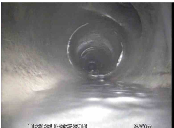
, 00:00:39, 3.08 m Junction at 1 o'clock, diameter: 100mm
