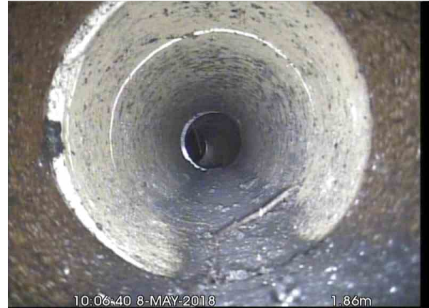
, 00:00:28, 1.86 m Crack, circumferential at joint from 12 o'clock to 12 o'clock
