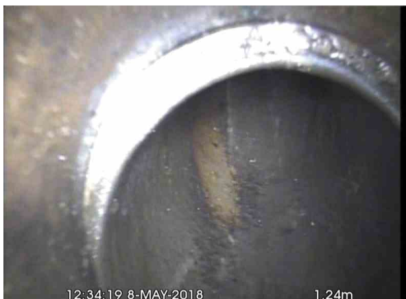
, 00:00:14, 1.24 m Joint displaced, medium
