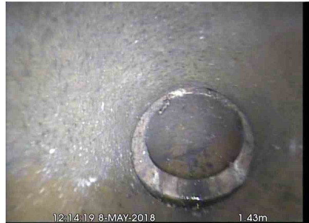
, 00:00:13, 1.43 m Joint displaced, medium
