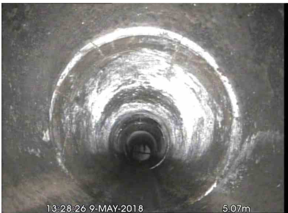
, 00:00:49, 5.07 m Cracks, multiple at joint from 9 o'clock to 3 o'clock
