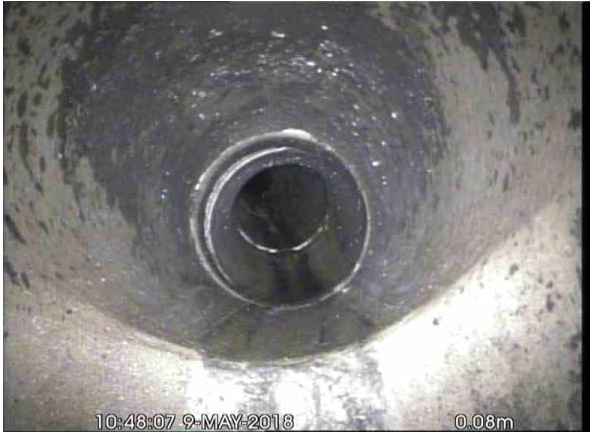
, 00:00:04, 0.08 m Junction at 6 o'clock, diameter: 150mm, External back drop
