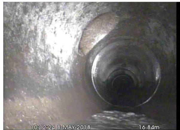
, 00:02:03, 16.76 m Junction at 10 o'clock, diameter: 100mm
