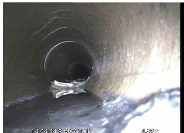
, 00:00:36, 4.99 m Settled deposits, other, 5% cross-sectional area loss, start
