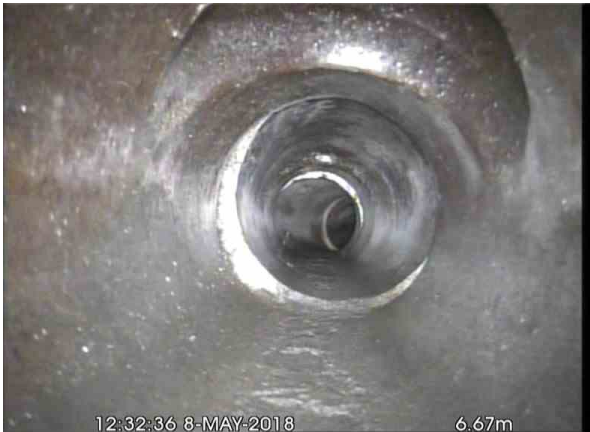
, 00:00:44, 6.67 m Junction at 1 o'clock, diameter: 100mm
