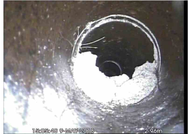
, 00:00:48, 2.96 m Attached deposits, other at joint from 4 o'clock to 8 o'clock, 35% cross-sectional area loss
