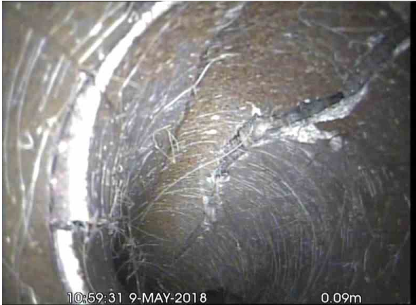
, 00:00:06, 0.09 m Fracture, multiple at joint from 12 o'clock to 12 o'clock
