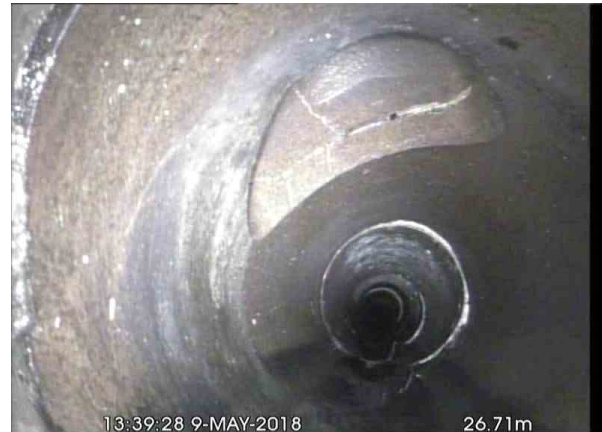
, 00:04:15, 26.71 m Defective junction, damaged at 10 o'clock, diameter: 100mm
