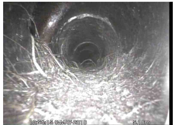
, 00:00:37, 5.18 m Junction at 10 o'clock, diameter: 100mm
