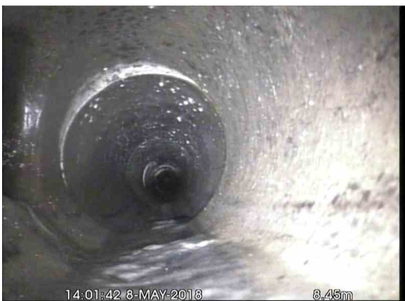
, 00:01:01, 8.45 m Junction at 9 o'clock, diameter: 100mm
