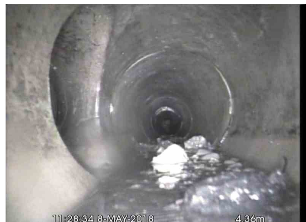
, 00:00:49, 4.36 m Junction at 9 o'clock, diameter: 100mm
