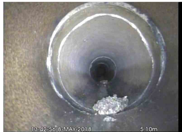
, 00:00:40, 5.10 m Crack, circumferential at joint from 12 o'clock to 12 o'clock
