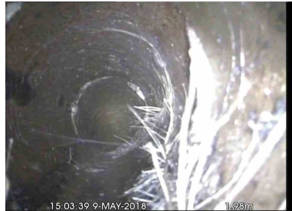
, 00:00:17, 1.98 m Roots, fine at joint
