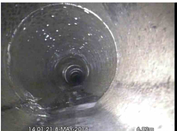
, 00:00:40, 6.03 m Roots, fine at joint
