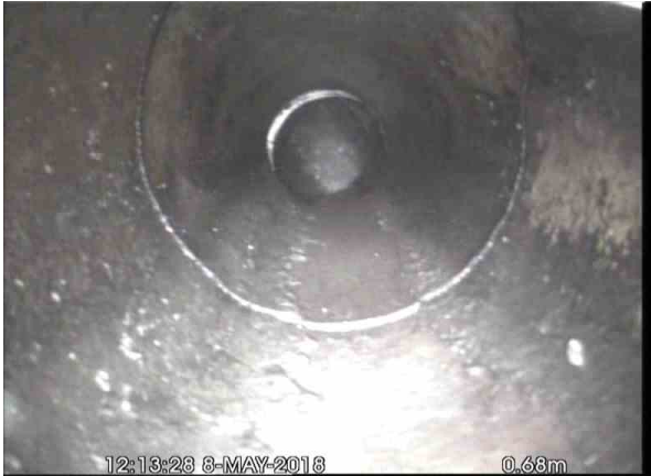
, 00:00:08, 0.68 m Crack, circumferential at joint from 12 o'clock to 12 o'clock
