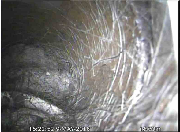
, 00:01:21, 16.70 m Collapsed drain or sewer
