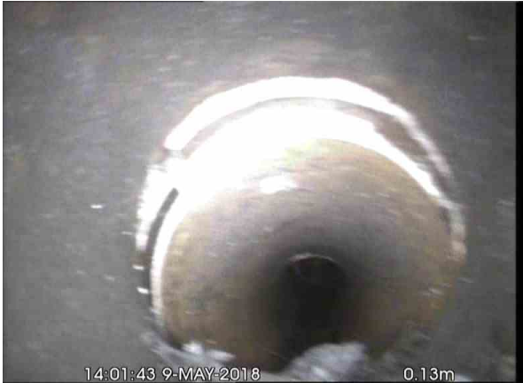
, 00:00:08, 0.13 m Fracture, multiple at joint from 10 o'clock to 2 o'clock
