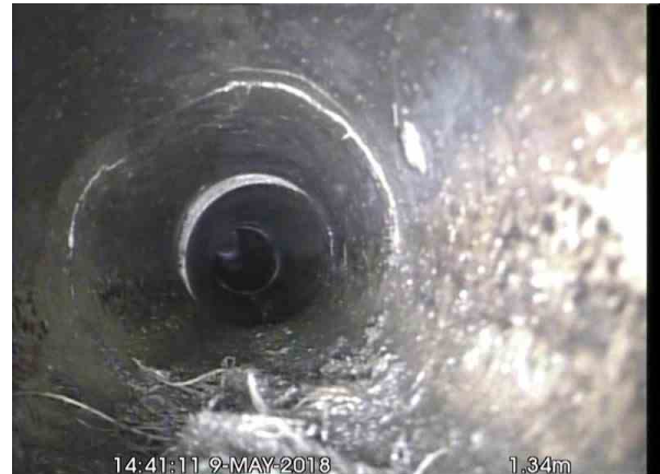
, 00:00:06, 1.34 m Crack, circumferential at joint from 12 o'clock to 12 o'clock
