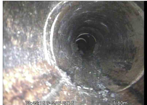
, 00:00:22, 2.00 m Crack, circumferential at joint from 8 o'clock to 12 o'clock
