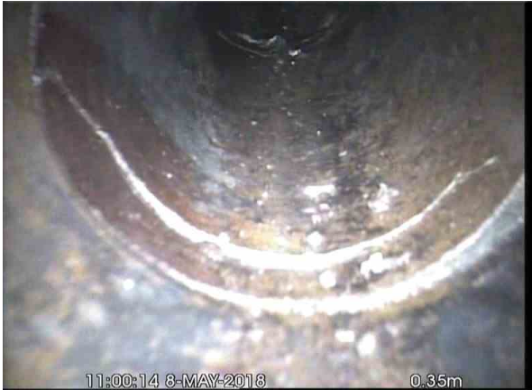
, 00:00:06, 0.22 m Crack, circumferential at joint from 5 o'clock to 8 o'clock
