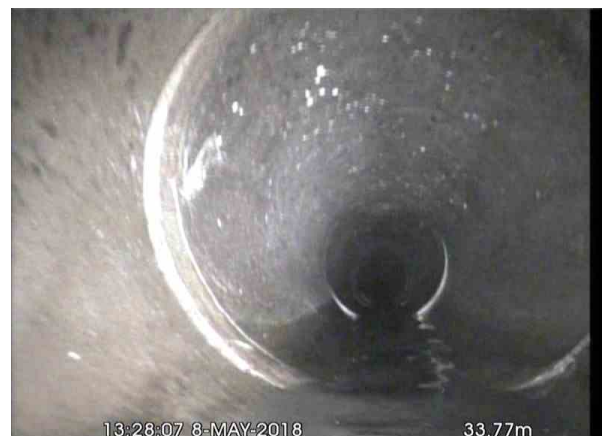
, 00:05:59, 33.77 m Crack, circumferential at joint from 7 o'clock to 10 o'clock
