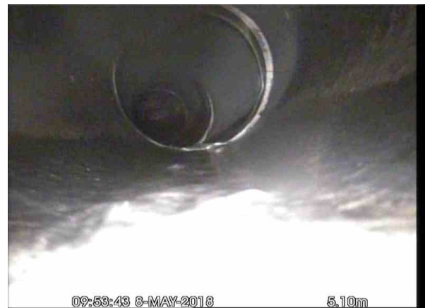
, 00:00:56, 5.10 m Crack, circumferential at joint from 12 o'clock to 6 o'clock
