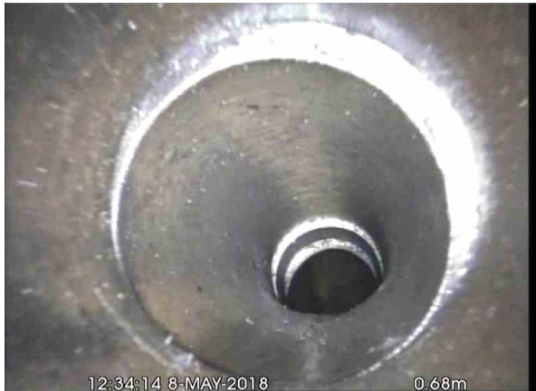
, 00:00:09, 0.68 m Joint displaced, medium
