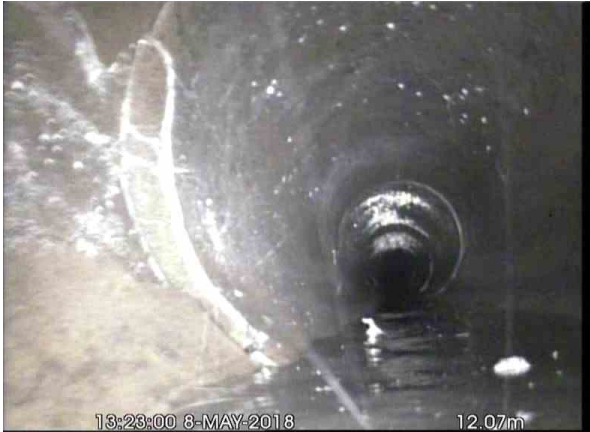
, 00:00:53, 12.07 m Fracture, circumferential at joint from 7 o'clock to 10 o'clock
