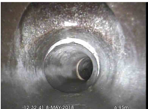
, 00:00:49, 6.95 m Junction at 12 o'clock, diameter: 100mm
