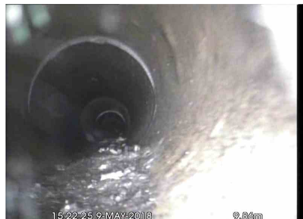
, 00:00:55, 9.86 m Settled deposits, fine, 5% cross-sectional area loss, start
