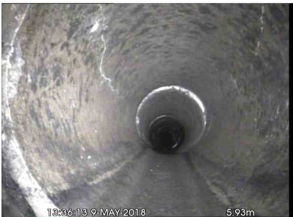
, 00:01:00, 5.93 m Crack, longitudinal at 11 o'clock
