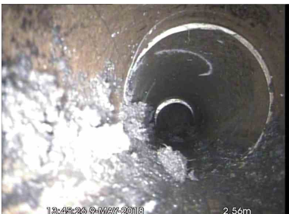
, 00:00:30, 2.56 m Crack, circumferential at joint from 9 o'clock to 2 o'clock
