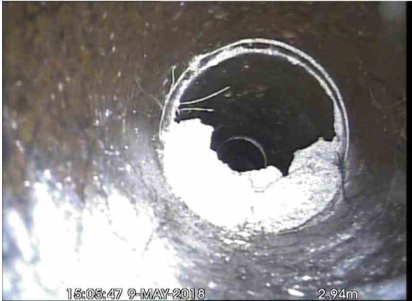
, 00:00:47, 2.94 m Crack, circumferential at joint from 12 o'clock to 12 o'clock
