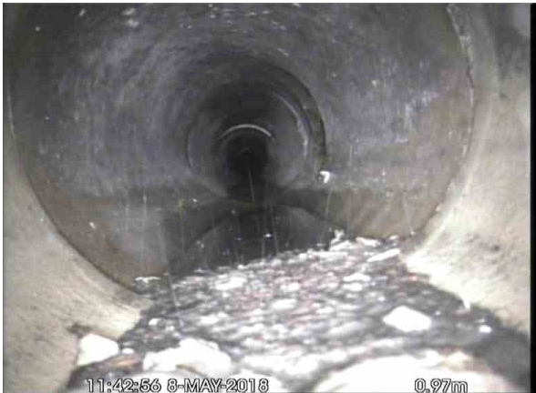
, 00:00:13, 0.97 m Settled deposits, other, 5% cross-sectional area loss
