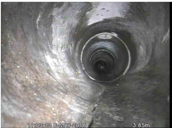
, 00:00:28, 3.85 m Fracture, longitudinal at 6 o'clock
