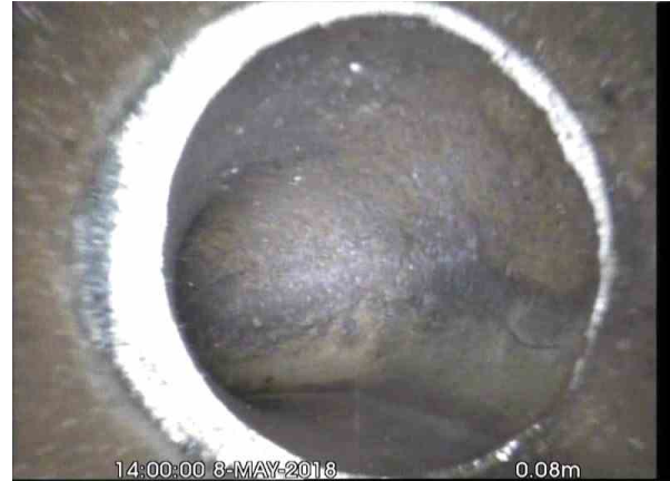
, 00:00:04, 0.08 m Joint displaced, medium
