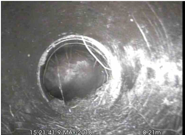
, 00:00:11, 0.21 m Roots, mass at joint, 5% cross-sectional area loss
