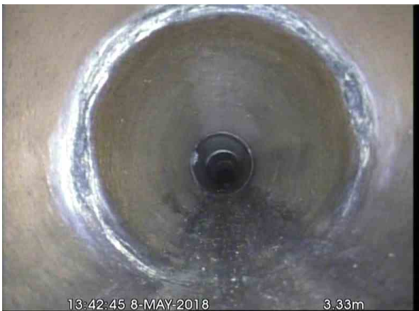
, 00:00:28, 3.33 m Attached deposits, other at joint from 12 o'clock to 12 o'clock, 5% cross-sectional area loss
