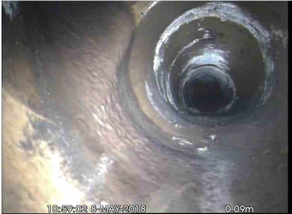
, 00:00:05, 0.09 m Junction at 10 o'clock, diameter: 100mm
