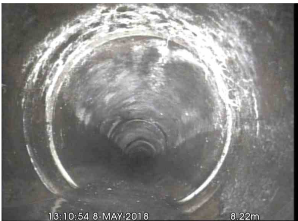
, 00:00:41, 8.22 m Crack, circumferential at joint from 12 o'clock to 12 o'clock
