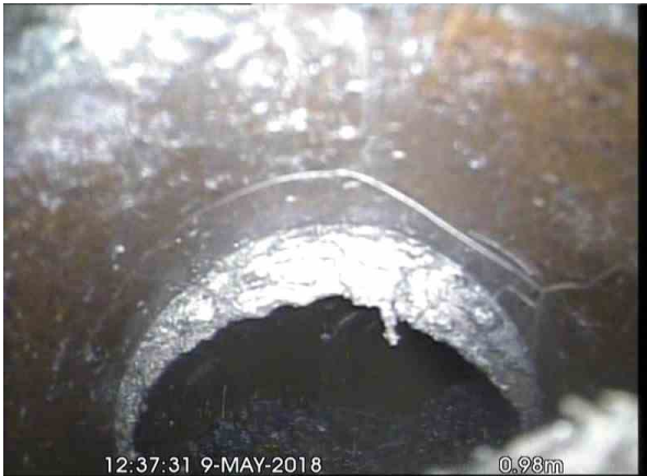
, 00:00:15, 0.98 m Joint displaced, medium
