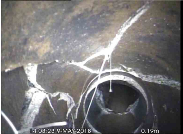
, 00:00:05, 0.19 m Broken pipe from 12 o'clock to 12 o'clock
