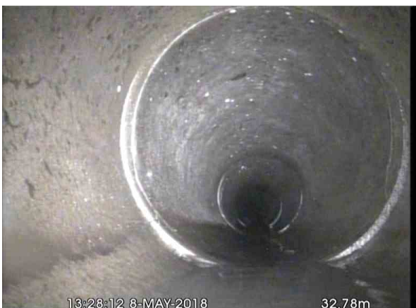
, 00:06:04, 32.78 m Crack, circumferential at joint from 7 o'clock to 4 o'clock
