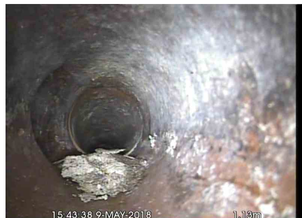
, 00:00:13, 1.13 m Junction at 9 o'clock, diameter: 100mm
