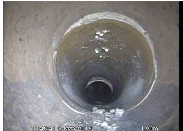
, 00:00:18, 1.90 m Crack, circumferential at joint from 3 o'clock to 9 o'clock
