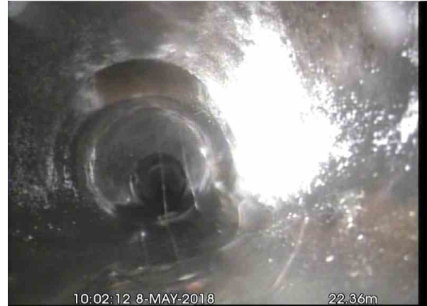
, 00:04:56, 22.36 m Junction at 1 o'clock, diameter: 100mm
