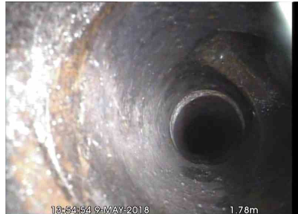
, 00:00:14, 1.78 m Junction at 2 o'clock, diameter: 100mm
