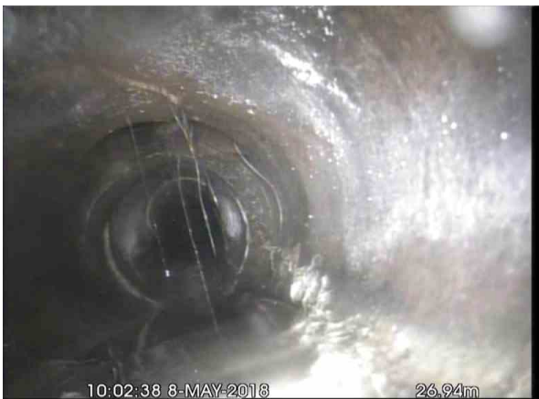
, 00:05:23, 26.94 m Junction at 1 o'clock, diameter: 100mm
