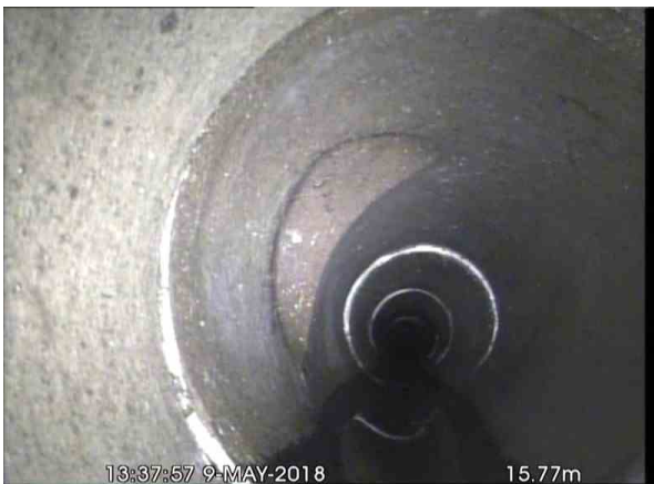
, 00:02:44, 15.77 m Junction at 10 o'clock, diameter: 100mm
