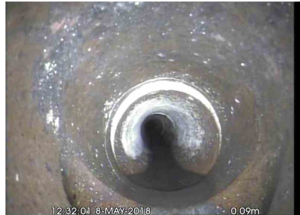
, 00:00:10, 0.09 m Crack, circumferential at joint from 7 o'clock to 2 o'clock
