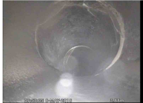
, 00:00:48, 3.88 m Cracks, multiple at joint from 9 o'clock to 3 o'clock
