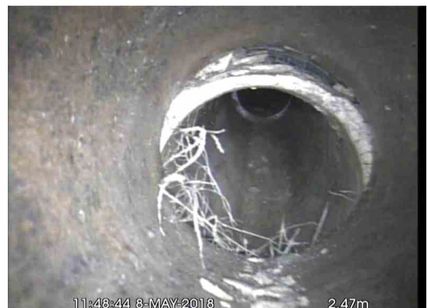
, 00:00:22, 2.47 m Roots, fine at joint
