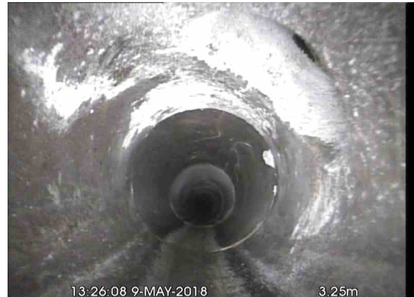
, 00:00:22, 3.25 m Junction at 1 o'clock, diameter: 100mm
