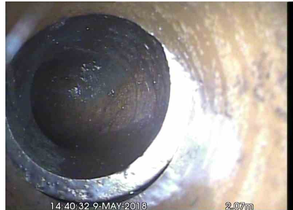
, 00:00:14, 2.07 m Joint displaced, medium
