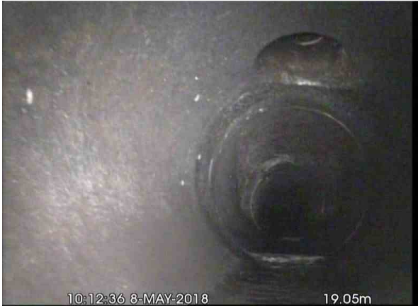
, 00:02:14, 19.05 m Junction at 1 o'clock, diameter: 100mm
