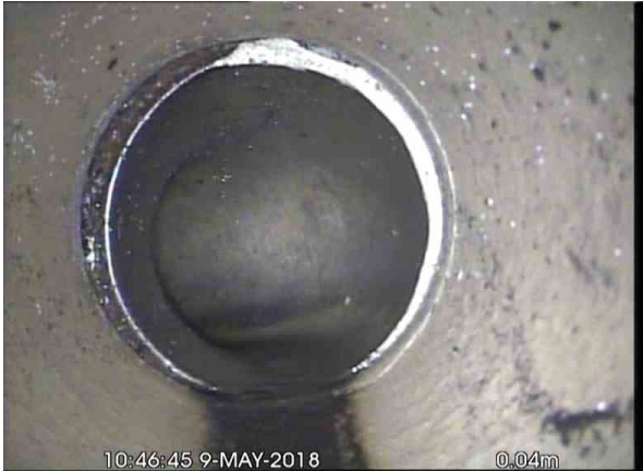
, 00:00:05, 0.04 m Crack, circumferential at joint from 12 o'clock to 6 o'clock
