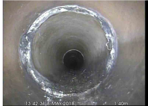
, 00:00:14, 1.40 m Attached deposits, other at joint from 12 o'clock to 12 o'clock, 5% cross-sectional area loss
