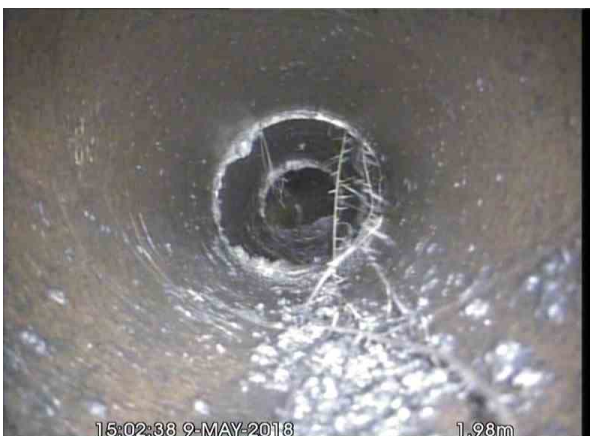
, 00:00:23, 1.98 m Roots, tap at joint
