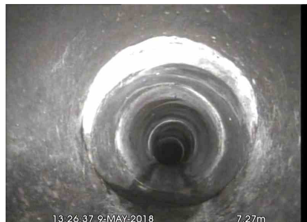
, 00:00:52, 7.27 m Joint displaced, medium
