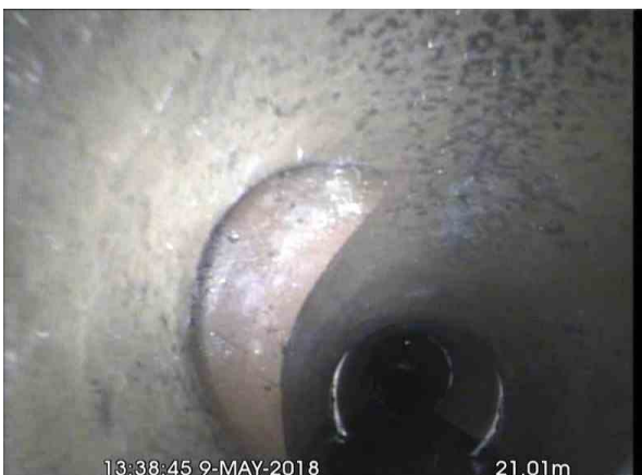
, 00:03:32, 21.01 m Junction at 9 o'clock, diameter: 100mm
