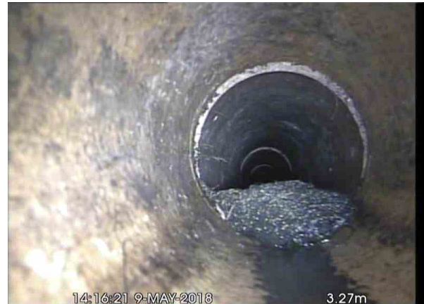
, 00:00:38, 3.27 m Roots, mass at joint, 10% cross-sectional area loss
