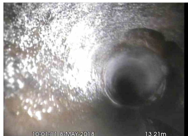
, 00:03:56, 13.21 m Junction at 1 o'clock, diameter: 100mm
