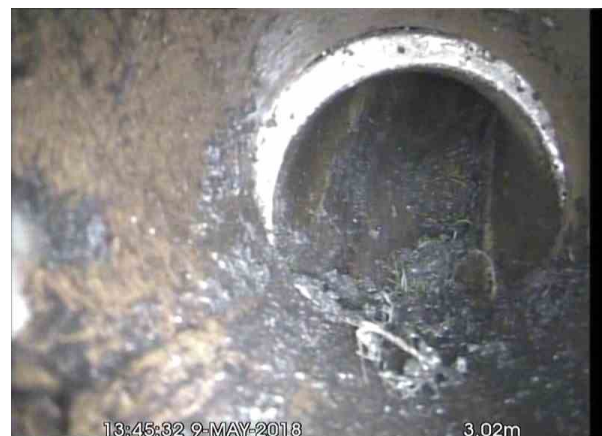
, 00:00:36, 3.02 m Joint displaced, medium
