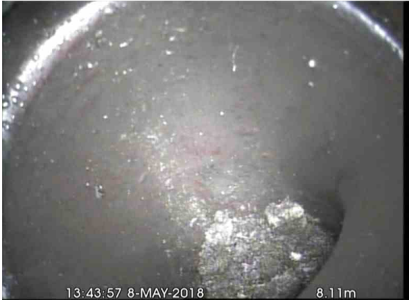
, 00:01:41, 8.11 m Settled deposits, fine, 30% cross-sectional area loss
