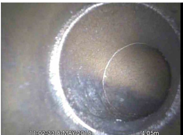
, 00:00:25, 4.05 m Crack, circumferential at joint from 12 o'clock to 12 o'clock
