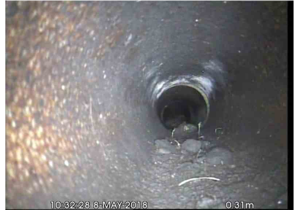
, 00:00:10, 0.31 m Settled deposits, fine, 5% cross-sectional area loss, start
