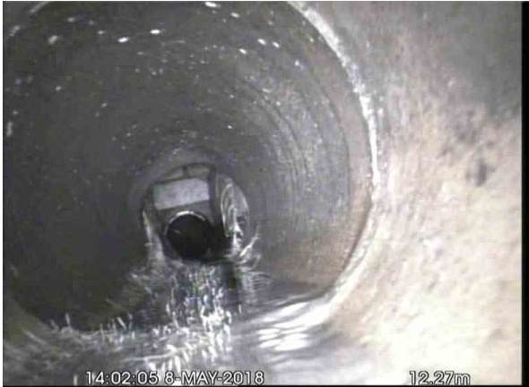
, 00:01:24, 12.27 m Roots, mass, 5% cross-sectional area loss
