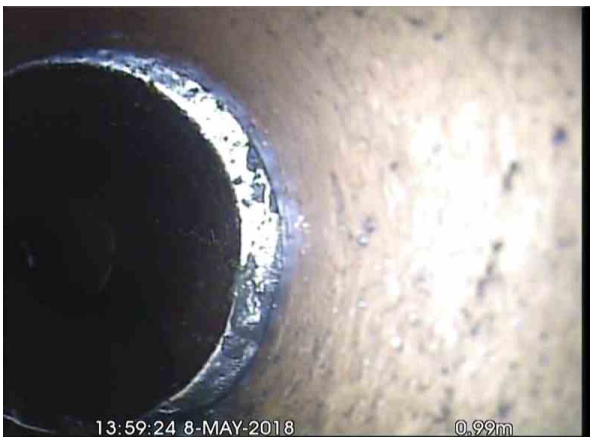
, 00:00:13, 0.99 m Joint displaced, medium
