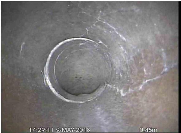
, 00:00:16, 0.45 m Fracture, longitudinal at joint at 4 o'clock
